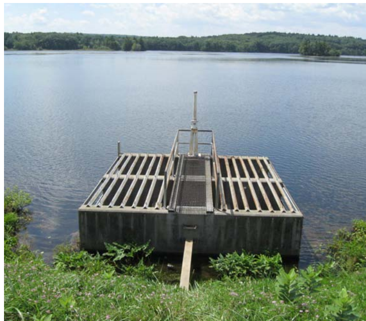
Spillway inlet at the George H. Nichols dam.
