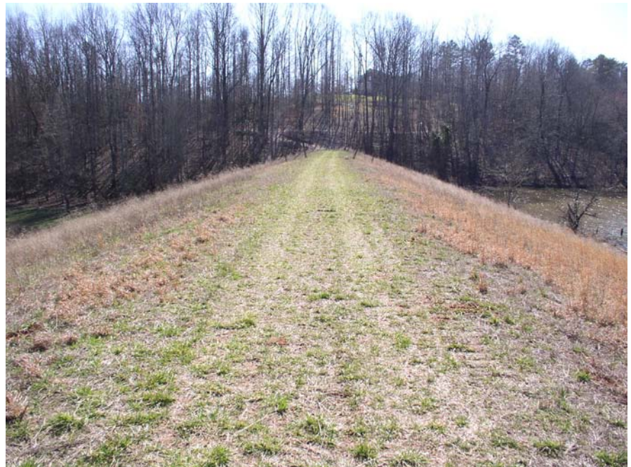
Sandy Creek Dam 23. Top of dam looking southeast. Vegetation has been maintained by mowing.
