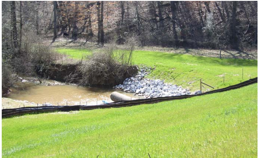
Sandy Creek Dam 15. Maintenance performed to reestablish vegetation on backslope and install riprap erosion protection on the principal spillway outlet basin.
