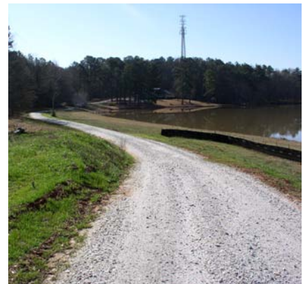
Marbury Creek Dam 22. Improvements to private road on top of dam (maintenance).
