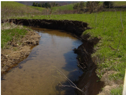
Before work began, this photo shows eroded streambank.
