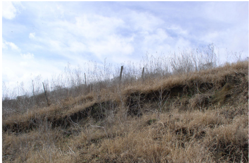
This slope slide on the Upper Brushy Creek Dam No. 29 will be repaired by removing the soil, treating with lime, and replacing to stabilize the slopes.
