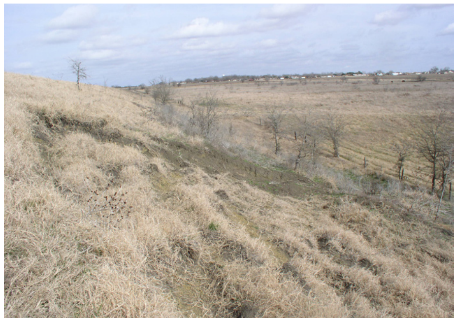
Soils have slid down the dam as a result of periods of heavy rainfall following extended drought.
