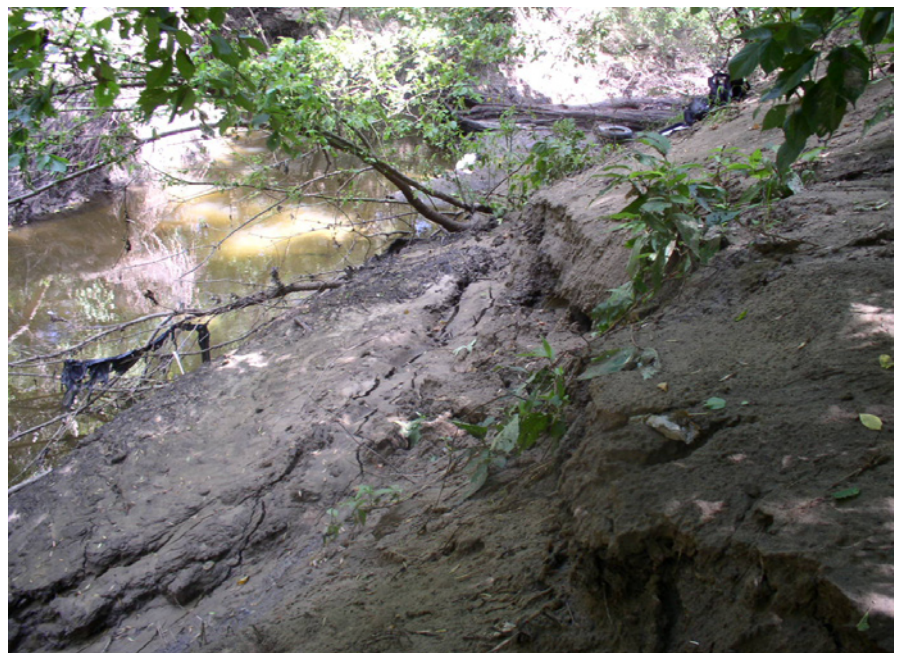
Establishing vegetation on these eroding stream banks will improve water quality.
