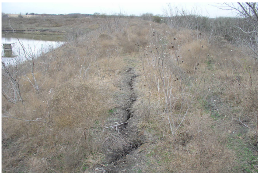
Periods of heavy rainfall following extended drought caused the soil to separate and slide.
