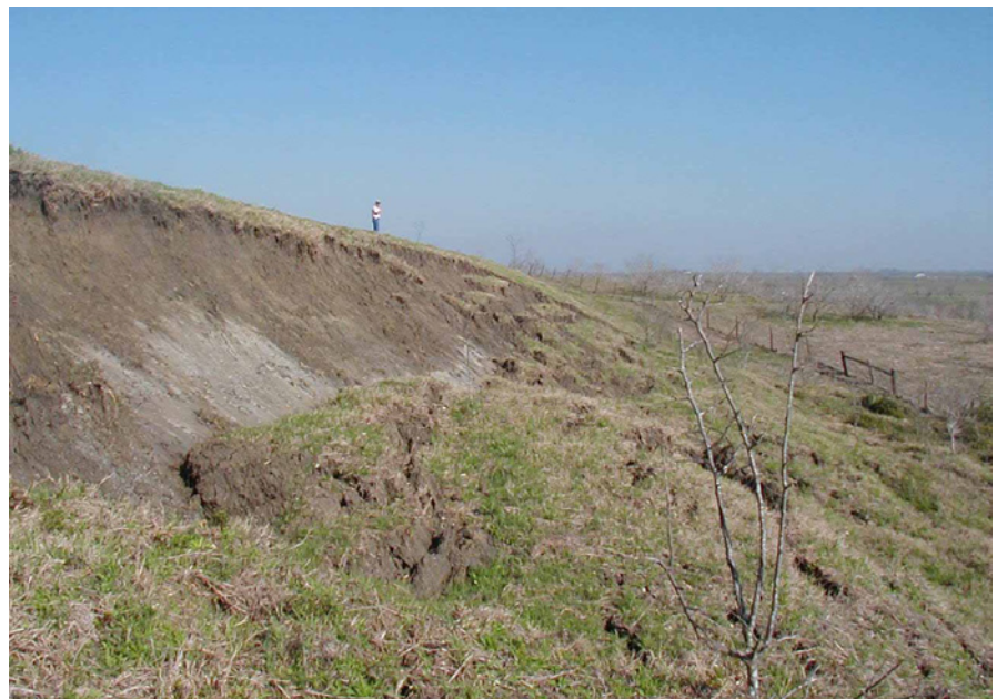
Slope slides on the dams will be repaired by removing the soil, treating with lime, and replacing to stabilize the slopes.
