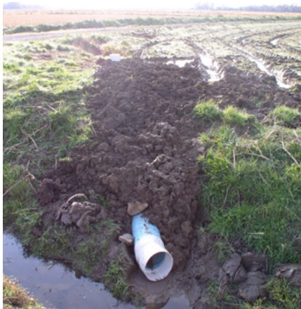
As seen above, a previously funded drop pipe water control structure.
