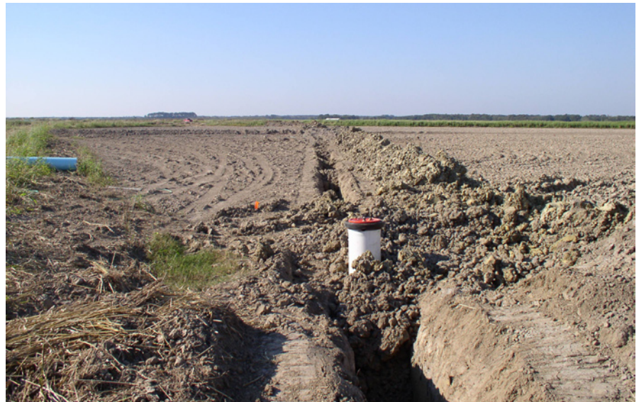
A previously funded irrigation underground pipeline installed for efficient use of water supply and fuel cost reduction.
