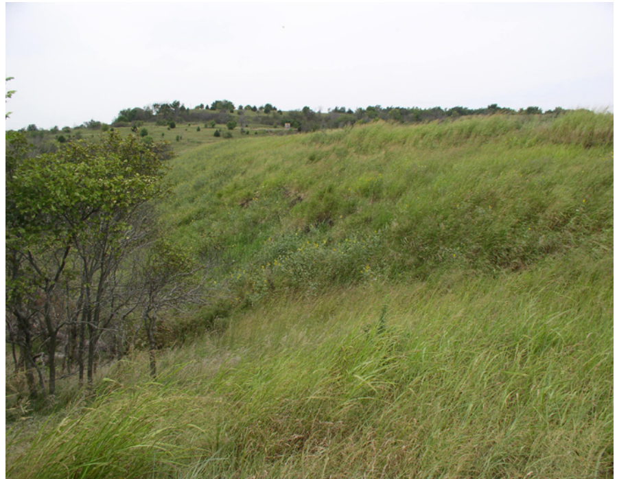
The downstream slope of the dam on Site 18 has experienced two slope failures since the fall of 2006.
