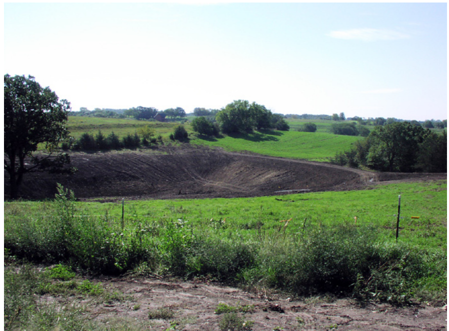
Construction was recently completed on this grade stabilization structure when this picture was taken in 2006.
