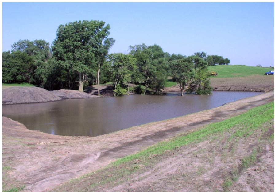
A newly constructed grade stabilization structure, completed in 2007, in the Hacklebarney Watershed with trees in the background that provide habitat for wildlife.
