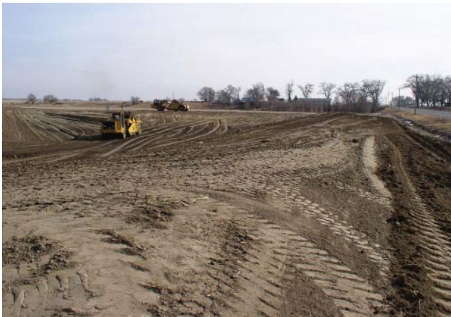
Preparation for mesh liner to be installed on a confined animal feeding operation to help prevent the leaching of nitrates and nutrients into groundwater.
