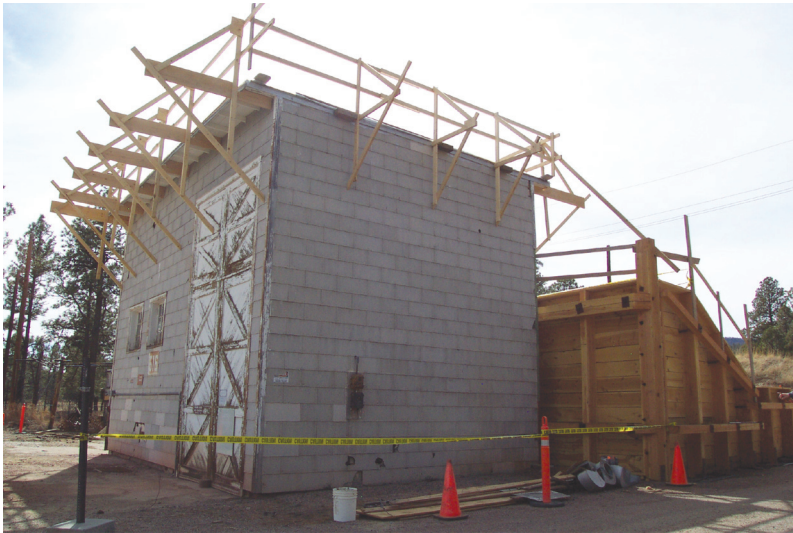
Phase 2 reconstruction of the assembly building roof (note reconstructed retaining wall at rear of building).
