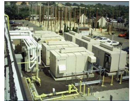
CHP system at telecom center
