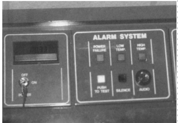
Figure 2 An alarm system that calls you or a guard if there is a temperature malfunction.
