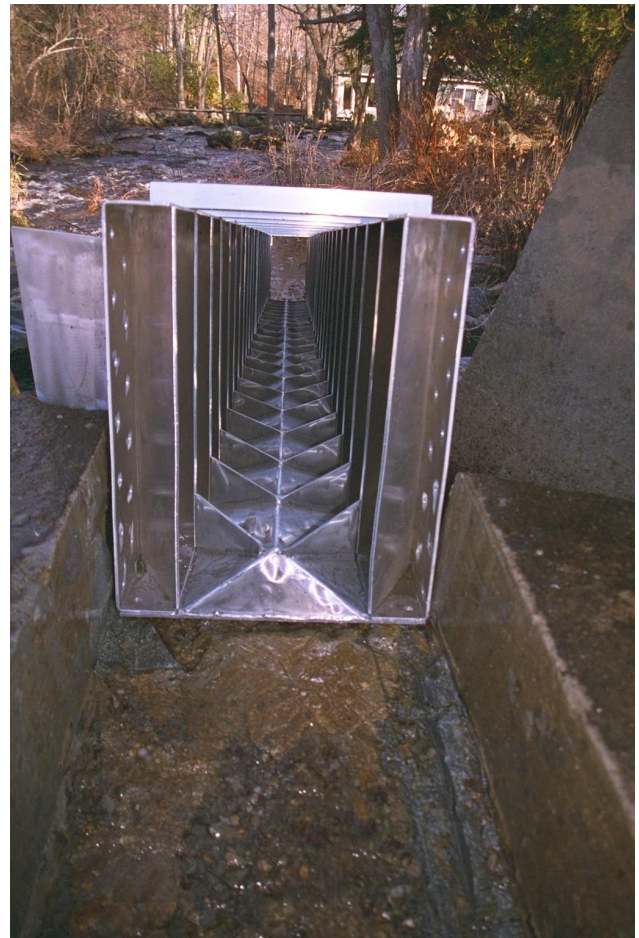
Fish bypass ladder installed on Parker River Dam, Byfield, MA, 2000. NOAA Restoration Center Community-based Restoration Project. Photo Credit: NOAA photo library.
