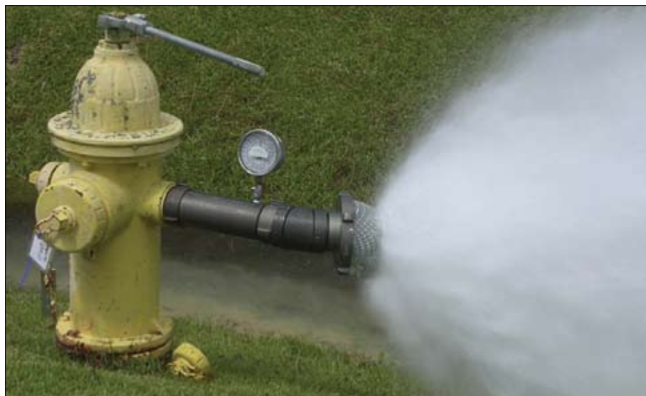
Figure 2. An integrated Pitot gauge and a wire-cage diffuser were installed on two flow hydrants.
