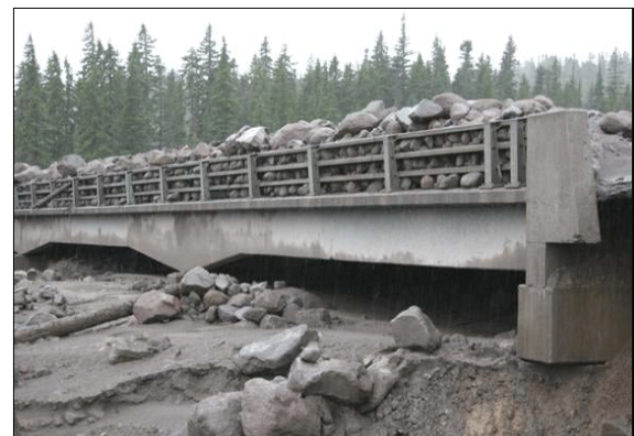
Aftermath of flooding and debris flow on the White River Bridge in Oregon. Photo courtesy: Doug Jones, Mt. Hood NF
