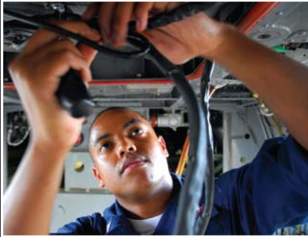
AE3 Christopher Houston, assigned to the "Blackjacks" of HSC-21, reattaches a distributor harness to the environmental-control system of an MH-60S Sea Hawk helicopter at Naval Air Station North Island. Navy photo by MC3 Joshua Valcarcel
