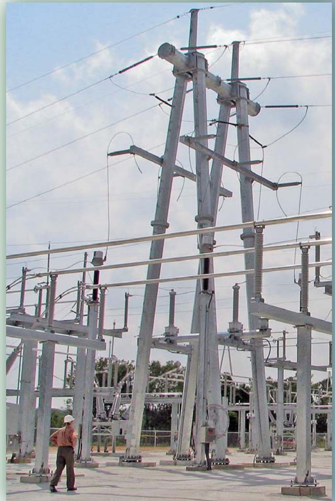
The Hilltop Interconnection was completed to improve regional transmission reliability in northwest Arkansas.
