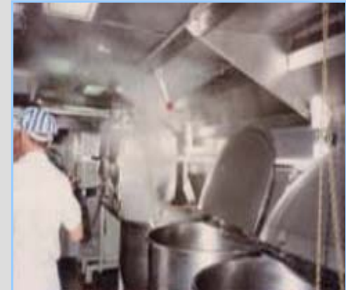
Controlling heat and humidity in shipboard galleys presents a design challenge.
