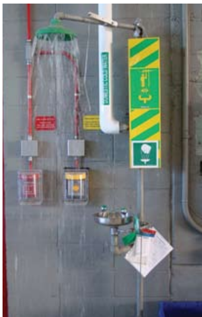
Water flows onto electrically hard-wired fire alarms
