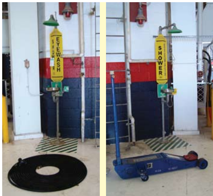
Blocked by trip hazards
