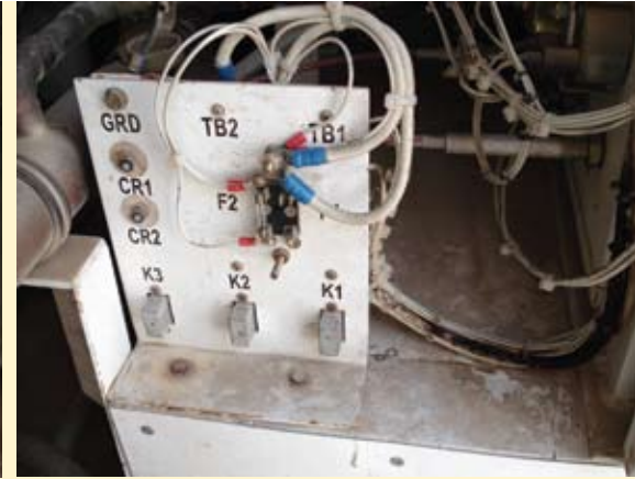
VP-8 bypassed fuse panel
