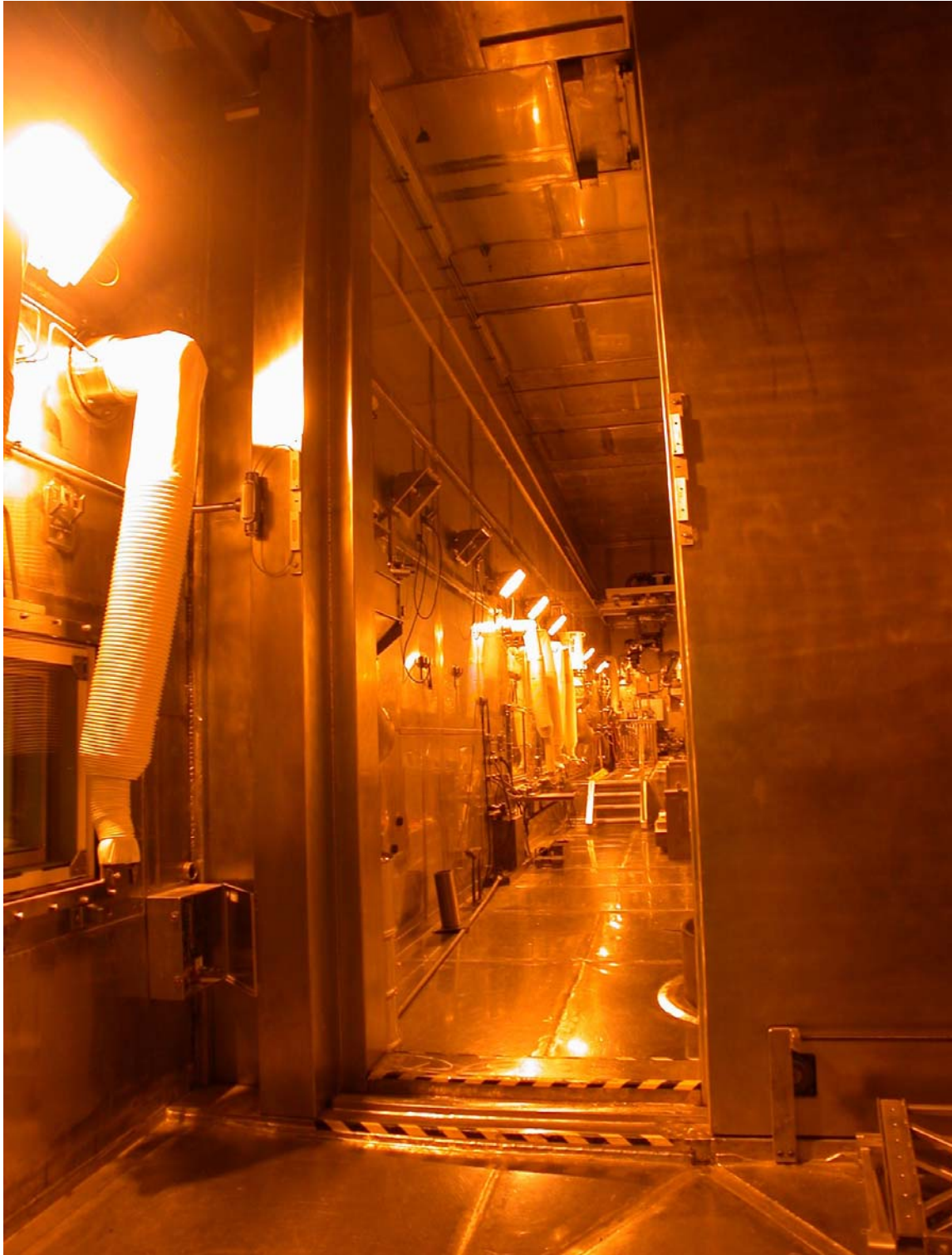
Fig. 5.2-57 View from transfer bay to maintenance bay.
