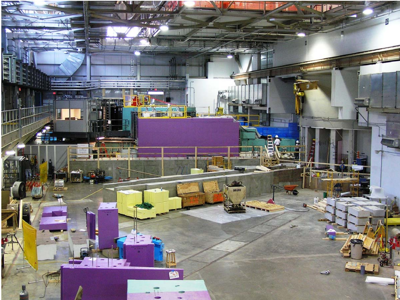
Fig. 5.5-18. Interior of the completed Target Building showing construction of the first four instruments.
