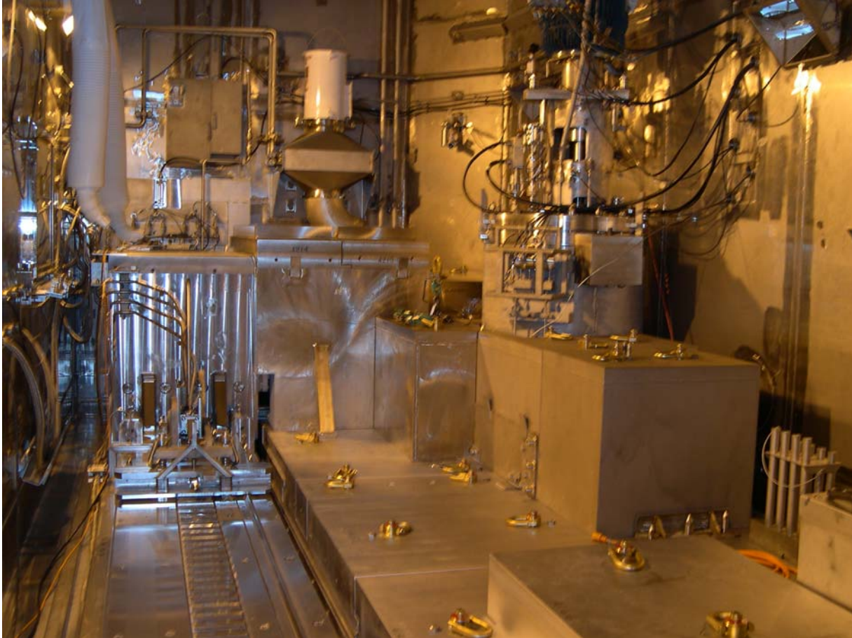
Figure 5.2-23. Target Service Bay with above floor shielding installed.
