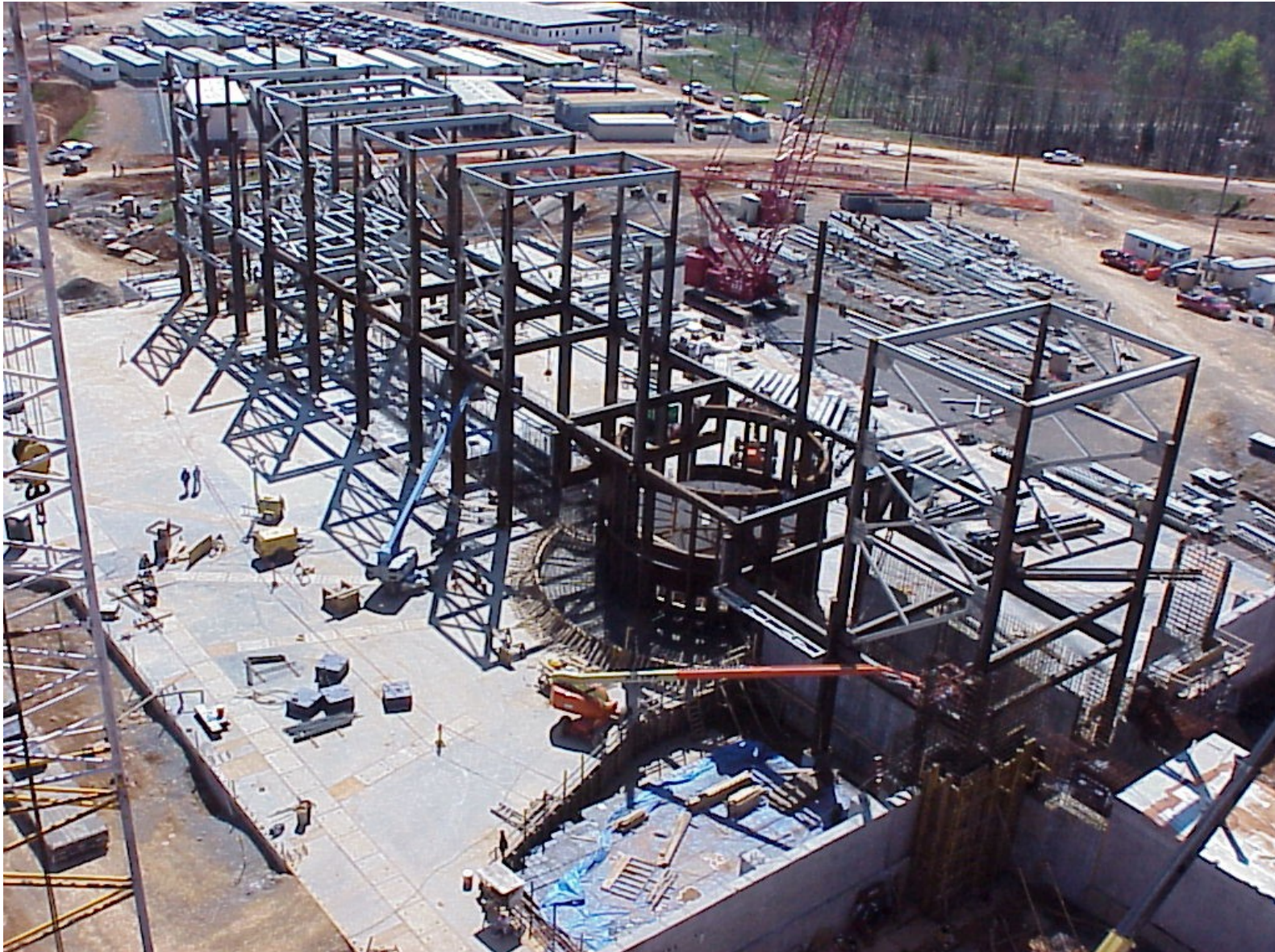
Fig. 5.5-15. Target Building construction as the target monolith and surrounding structure are installed.
