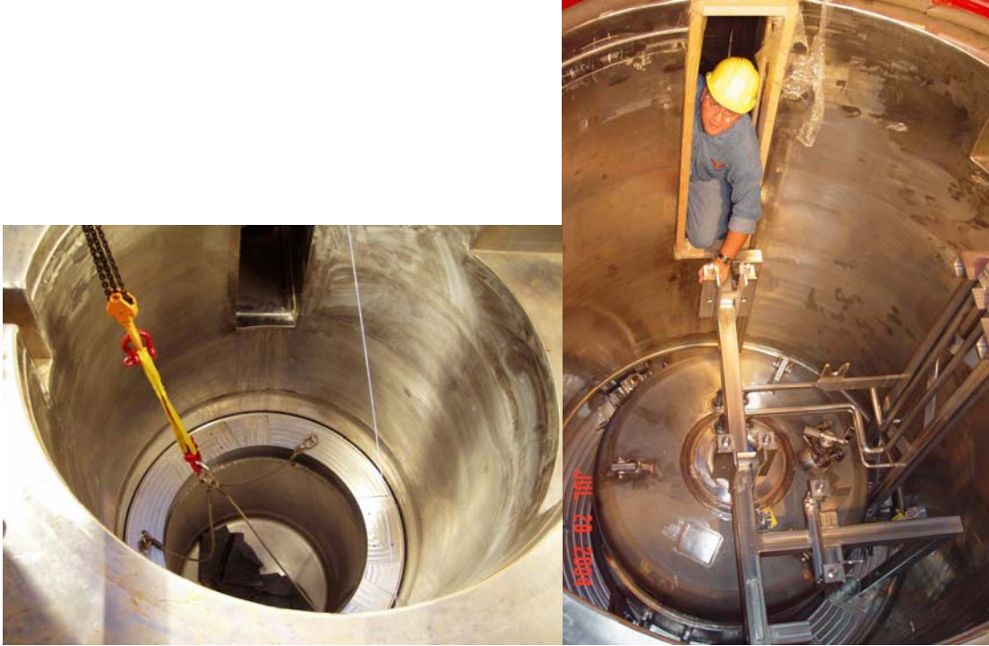
Fig. 5.2-21. Mercury collection basin and mercury storage tank installed in collection basin.
