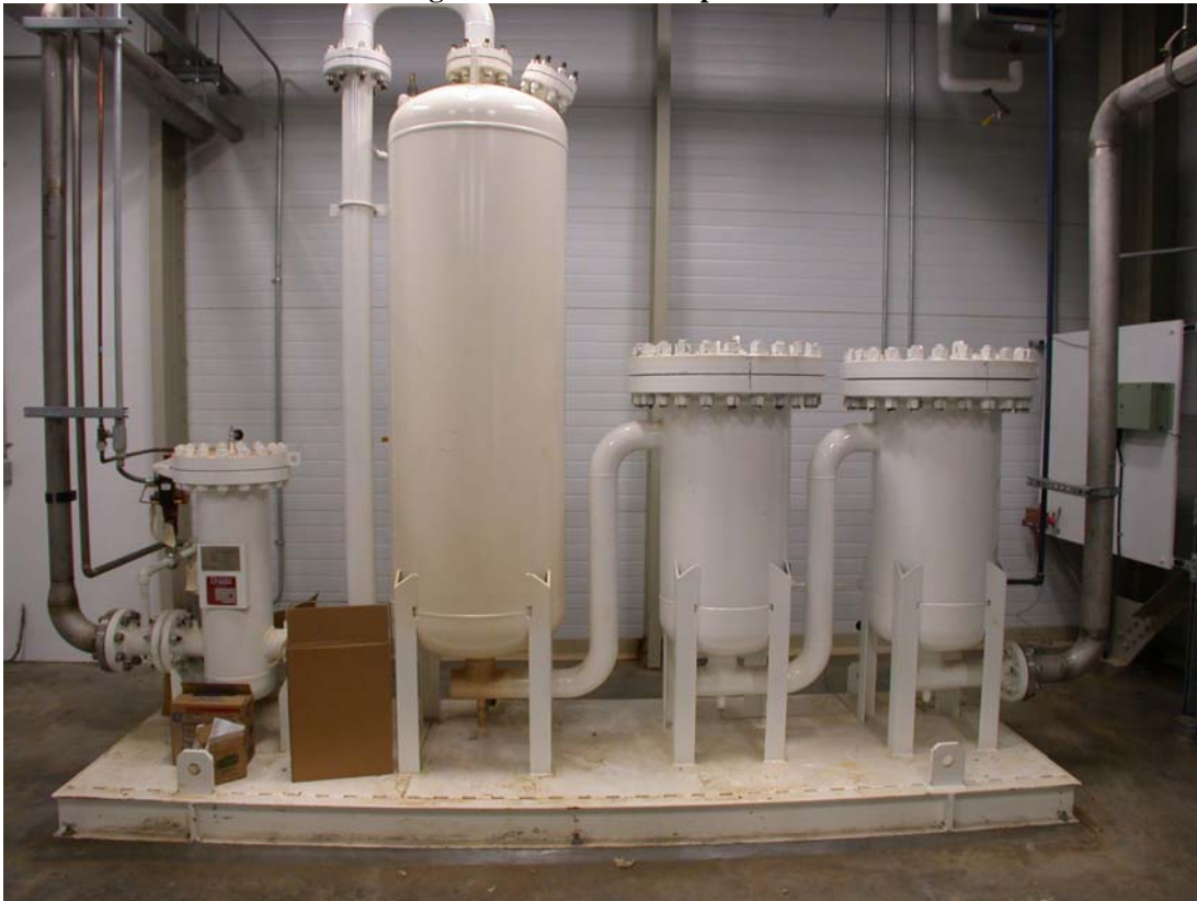
Fig. 5.2-41. Oil removal skid for helium compressor system.
