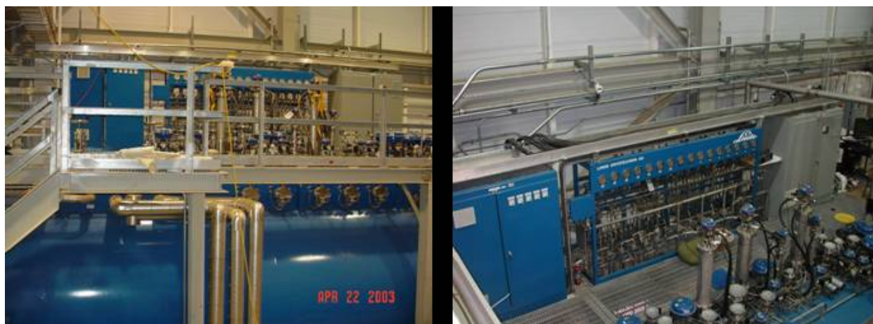
Fig. 5.1-14. The 4.5-K cold box (left) and associated controls (right) in the CHL Building feeding the liquid helium into the transfer line.
