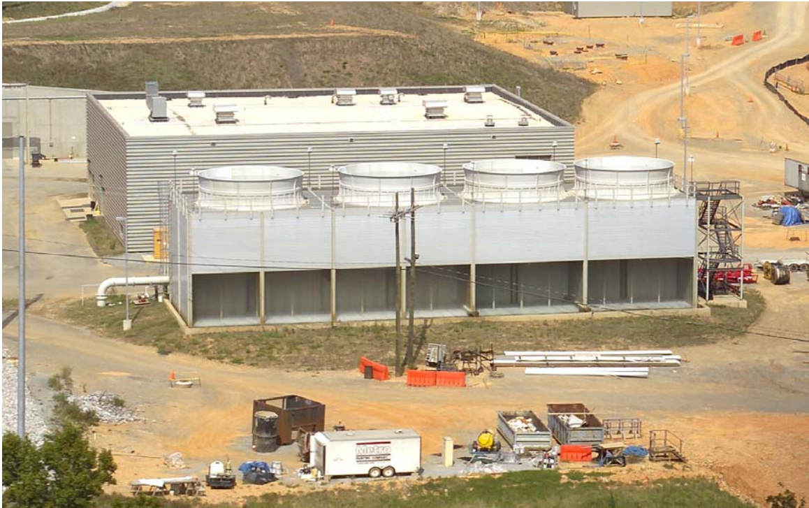
Fig. 5.5-24. Aerial view of the Central Utility Building and central cooling tower.
