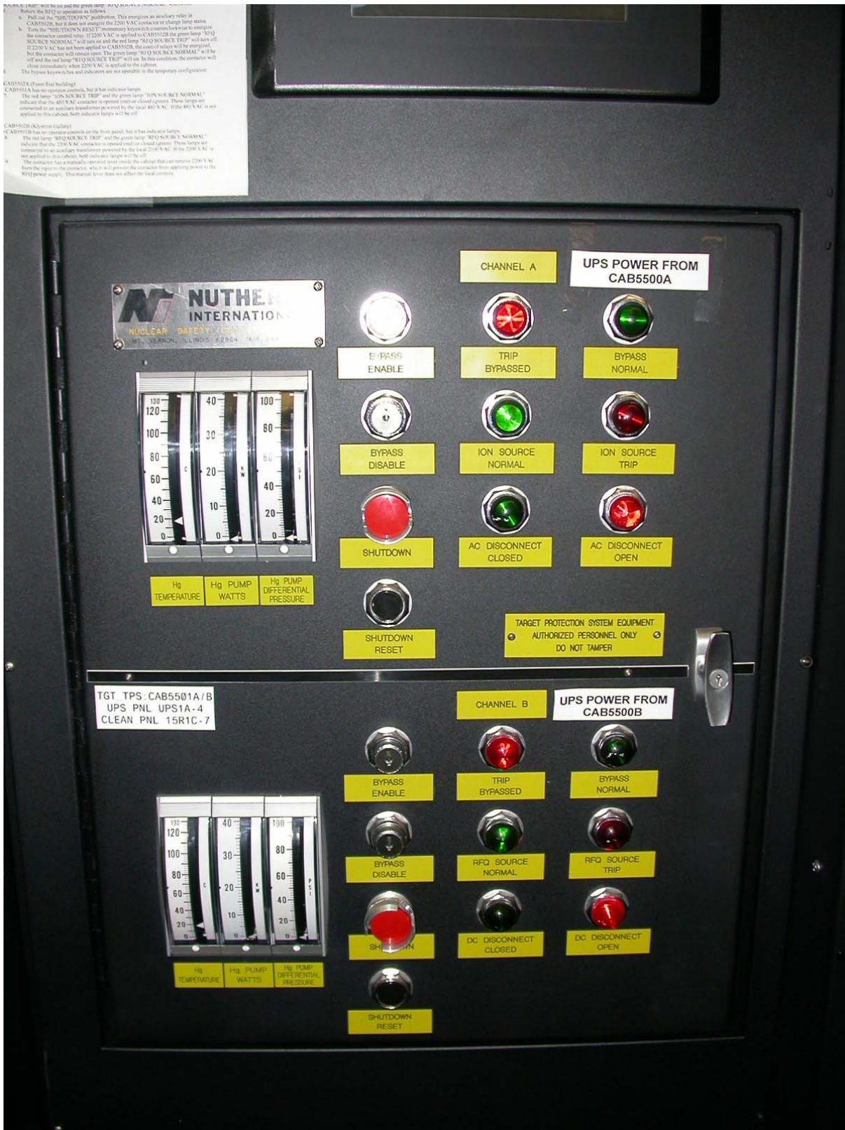
Fig. 5.2-84.. TPS cabinet CAB5501A/B located in the Central Control Room.
