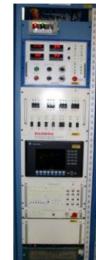
EQUIPMENT CONTROL RACK
