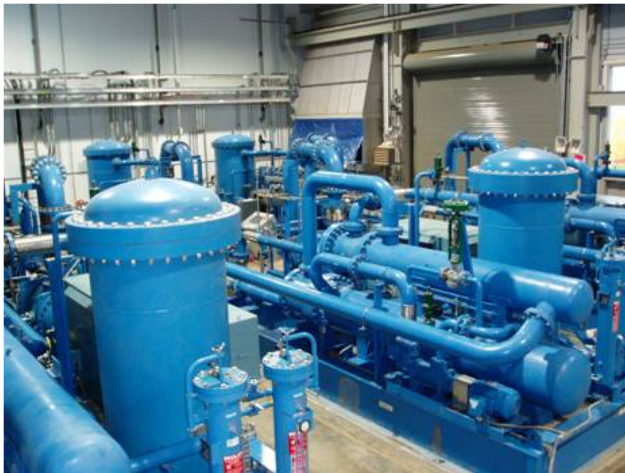
Fig. 5.1-13. Warm compressor installation in the CHL Building feeding into the 4.5-K cold box.
