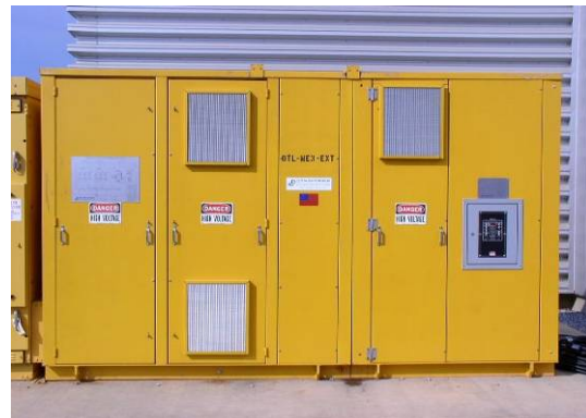
RECTIFIER TRANSFORMER AND FILTERS
