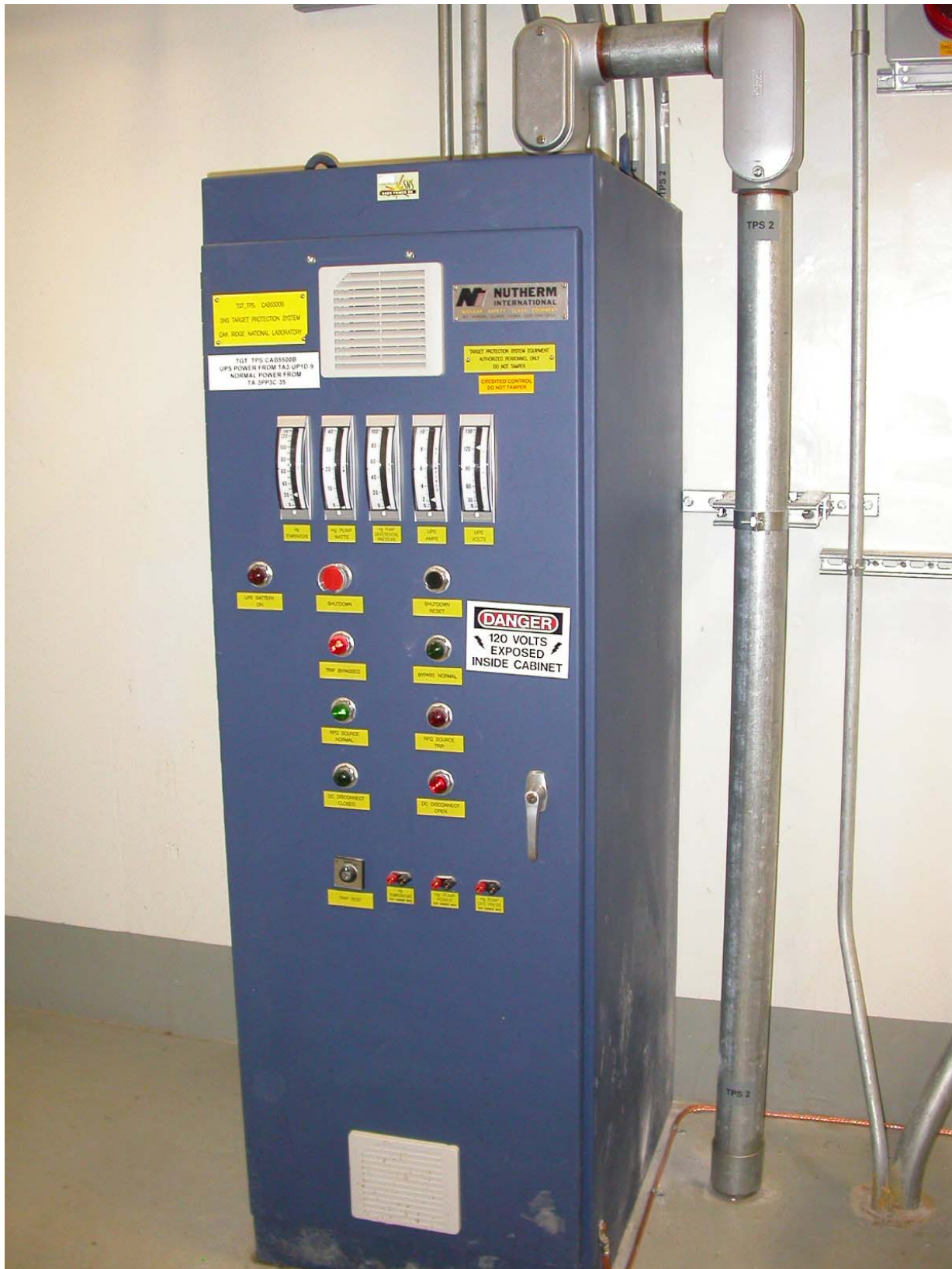
Fig. 5.2-83. TPS CAB5500B located in the Target Building service gallery.
