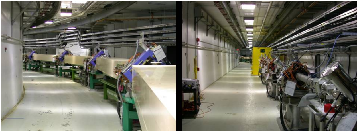
Fig. 5.1-22. Tunnel enclosure of the HEBT arc (left) and the beam transport from the linac to the arc (right). The beam is transported into the injection straight section of the ring.
