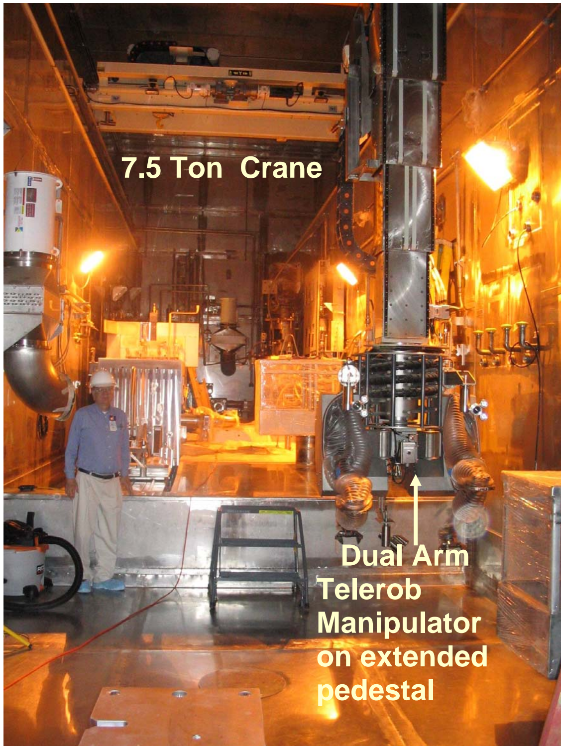
Fig. 5.2-69. Target service bay with manipulator and 7.5-ton crane.
