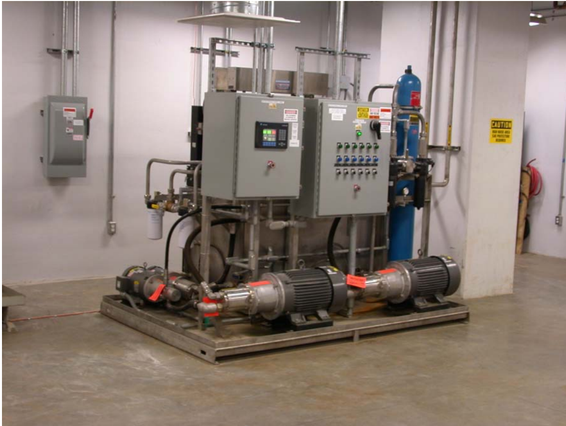
Fig. 5.2-51. Hydraulic power unit for the shutter drive system.
