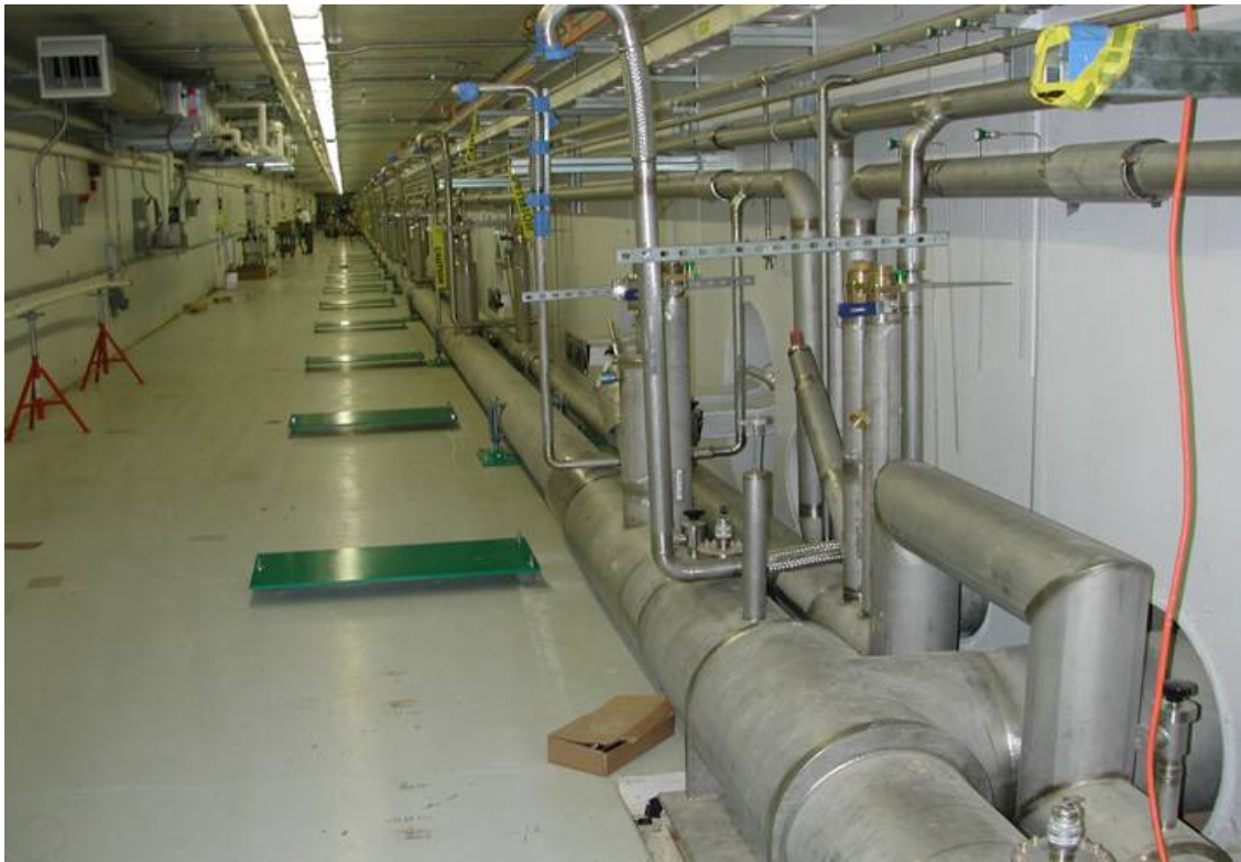
Fig. 5.1-12. Cryogenic transfer line in the linac tunnel all the way to the end of the additional nine cryomodules that are foreseen for a future power upgrade.
