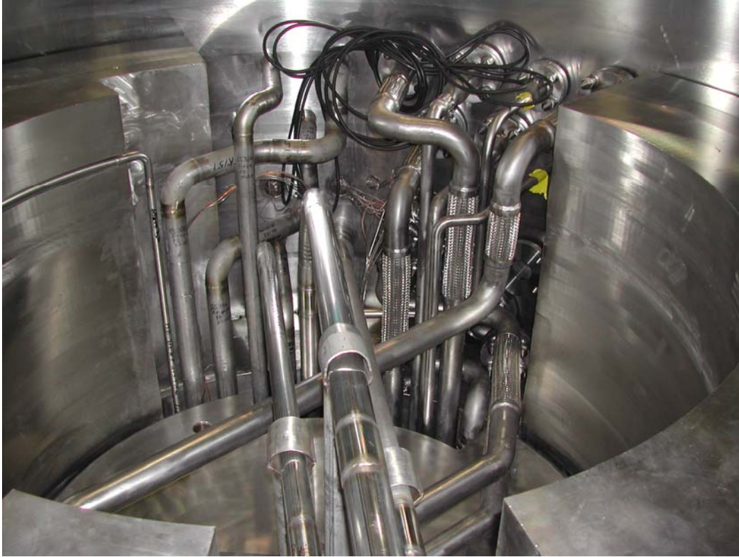
Fig. 5.2-32. Inner reflector plug installed with water lines connected, and transfer lines welded.
