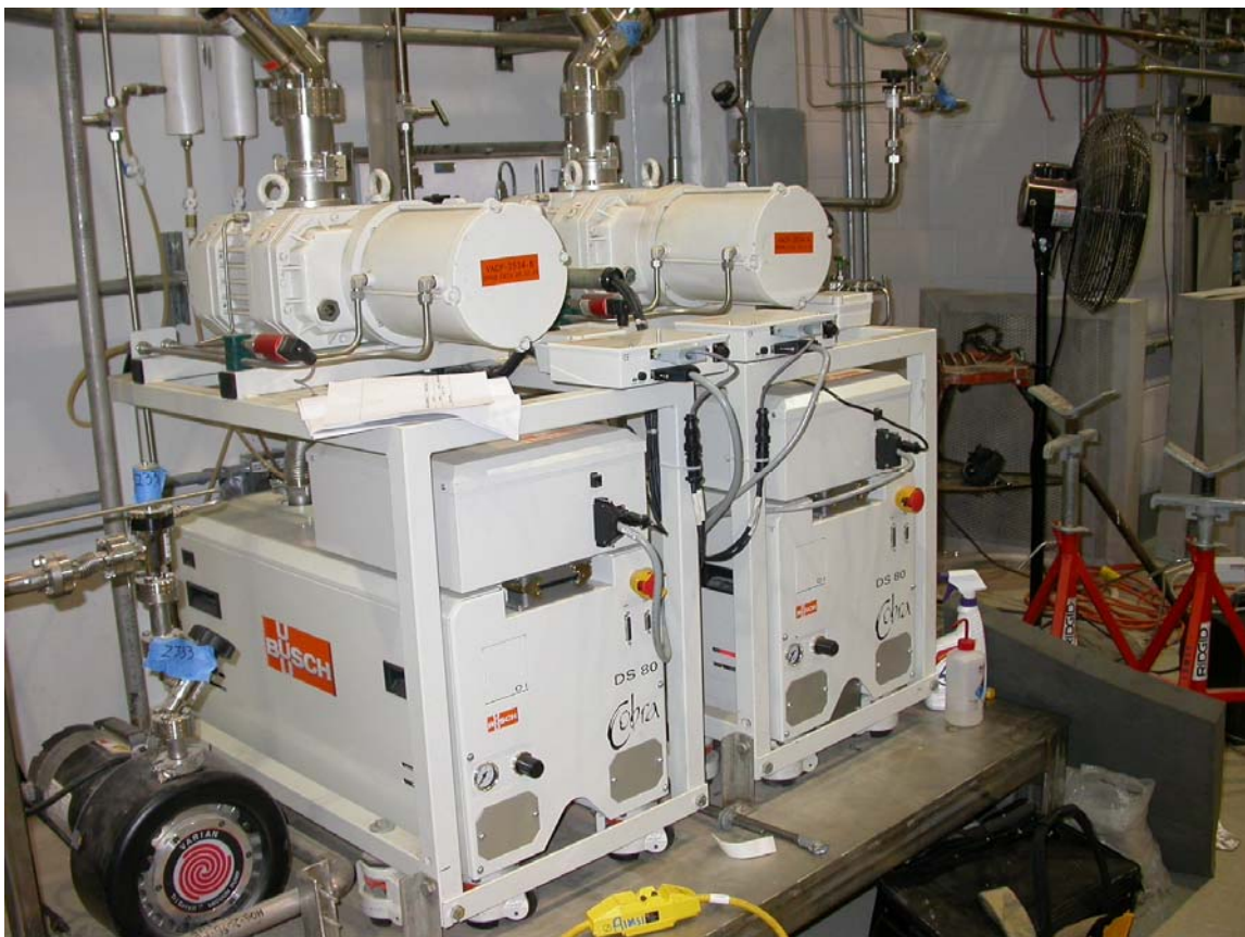
Fig. 5.2-79. Core vessel vacuum pumps.
