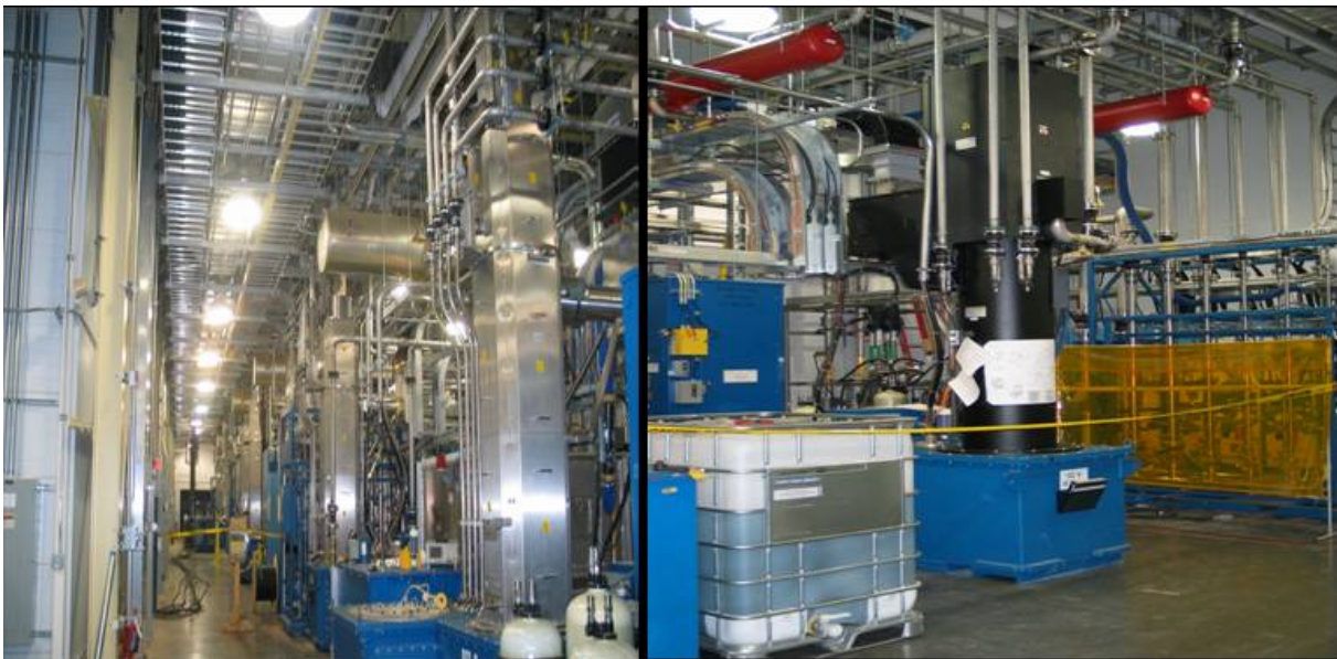
Fig. 5.1-7 The first part of the klystron gallery accommodates the 402.5-MHz klystrons and the associated support systems (left), followed by four 805-MHz klystrons driving the CCL (right).
