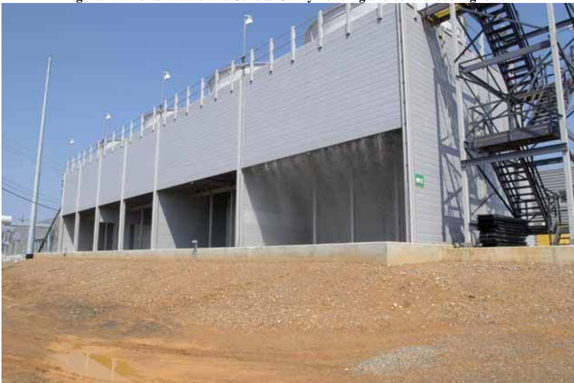
Fig. 5.5-25. Northward view of the central cooling tower.
