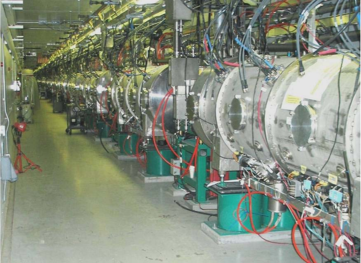
Fig. 5.1-16. View of the superconducting linac with a total of 23 cryomodules installed. The transfer line shown in Fig. 5.1-12 is behind the modules.
