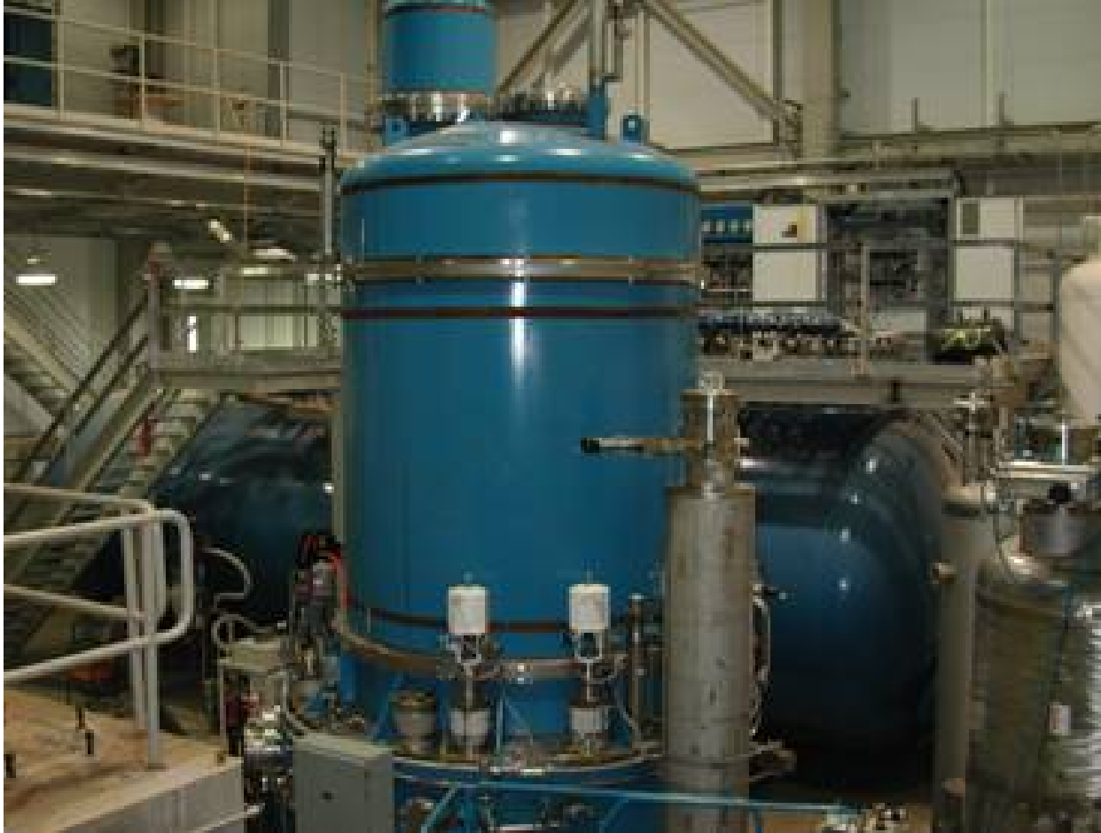
Fig. 5.1-15. Massive 2-K cold box in the CHL Building pumping down the transfer line to 40 mbar, allowing the generation of 2-K superfluid helium in the cryomodules.
