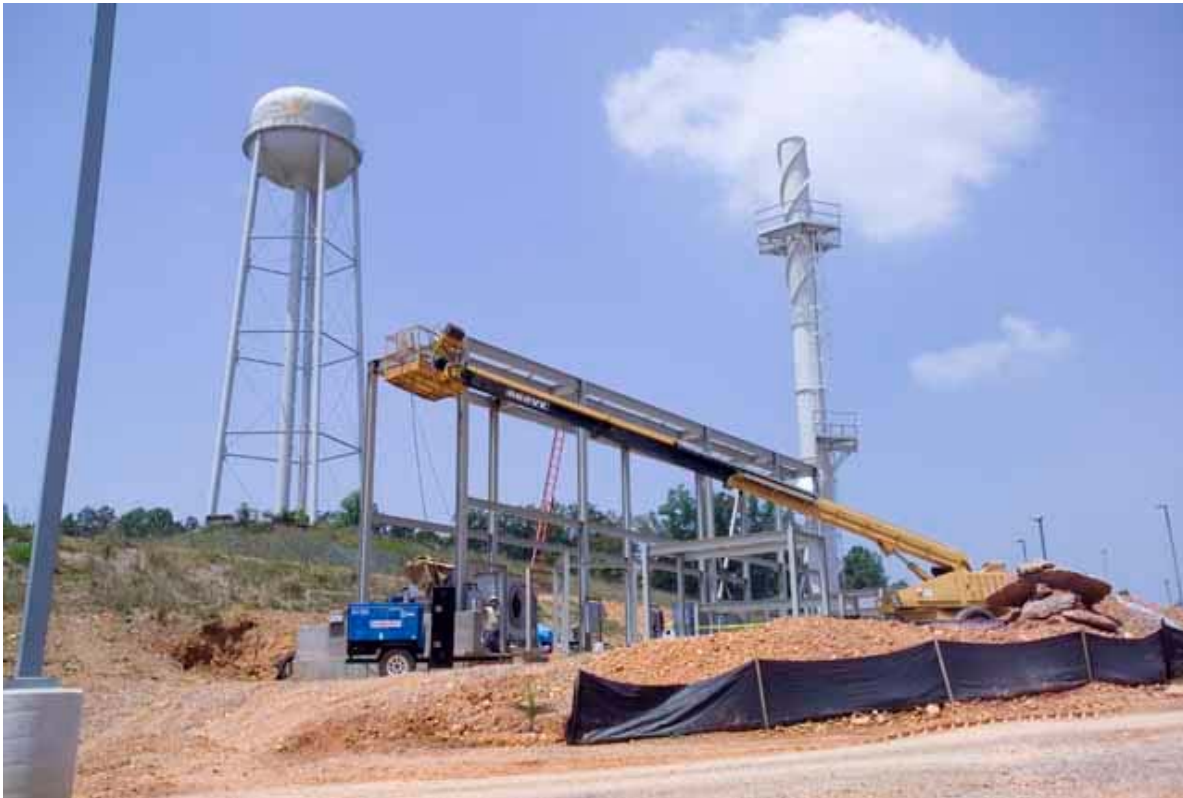
Fig. 5.5-27. Central exhaust facility.
