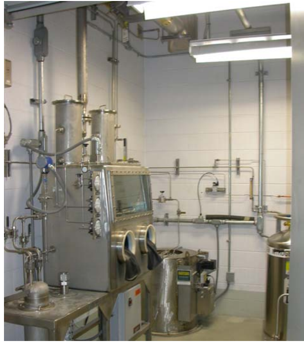
Fig. 5.2-82. MOTS after installation complete.
