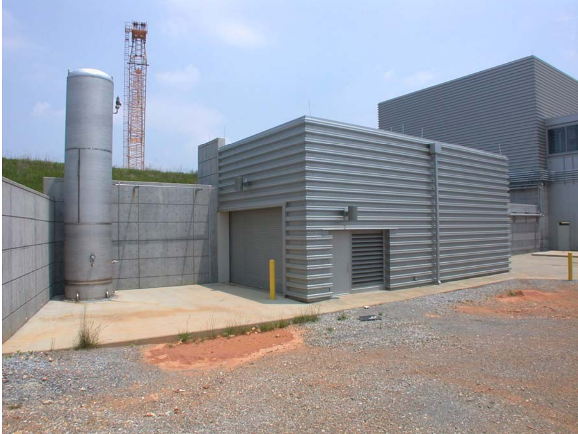
Fig. 5.2-38. Compressor Building and helium buffer tank to left.
