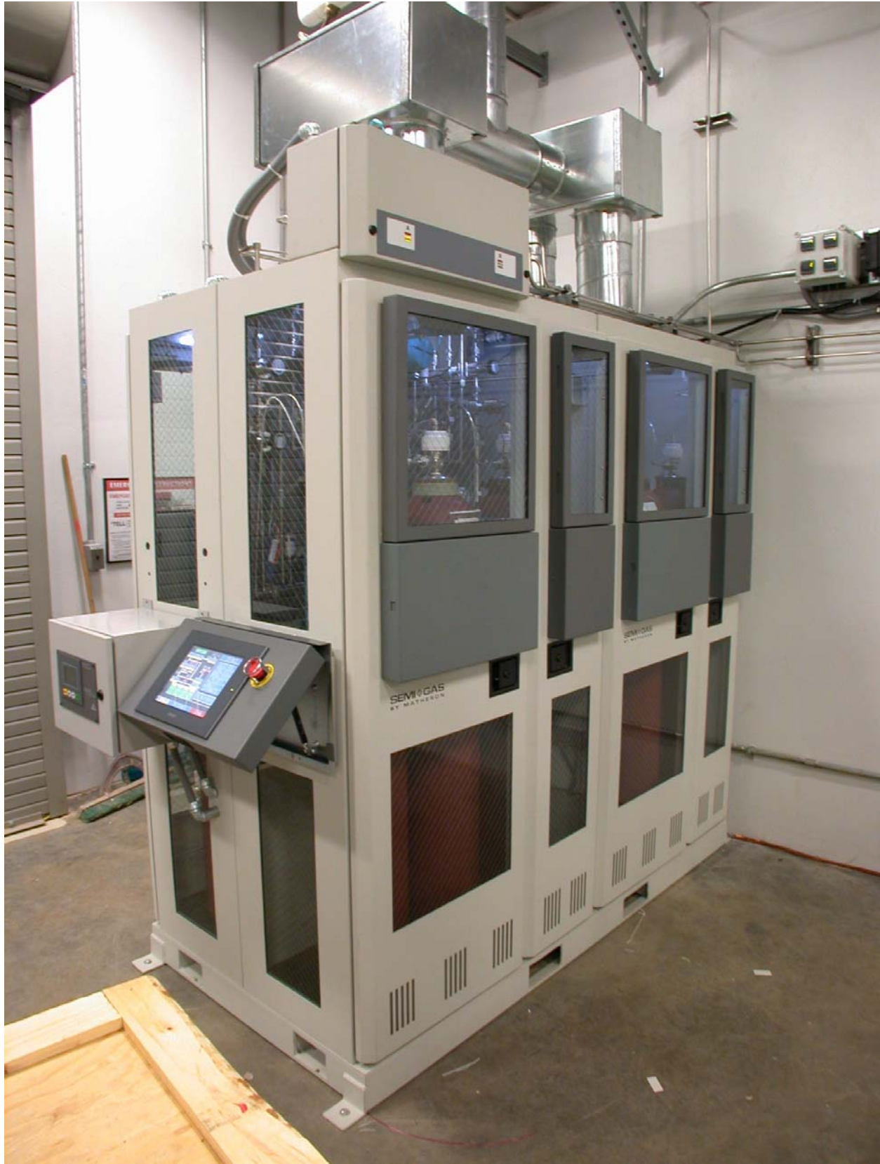
Fig. 5.2-39. Hydrogen gas cabinet in Compressor Building.
