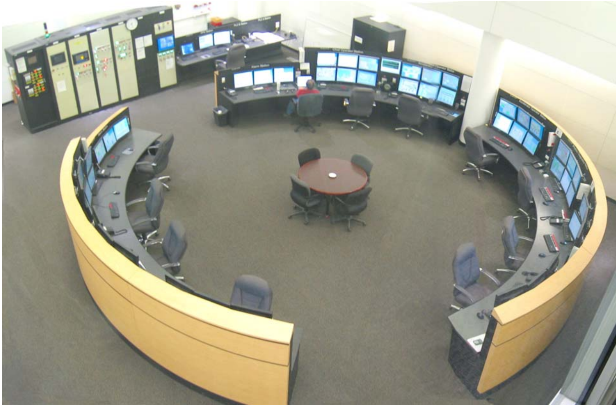
Fig. 5.4-3. Central Control Room.
