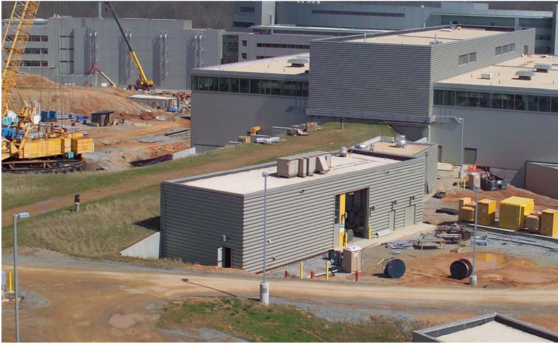
Fig. 5.5-8. Aerial view of the RTBT Service Building. The RTBT Service Building is on the left in front of the Target Building.
