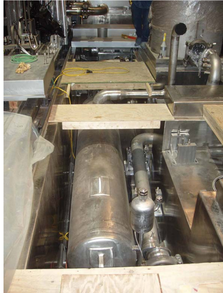
Fig. 5.2-13. Mercury double wall heat exchanger on tooling and installed in target service bay.
