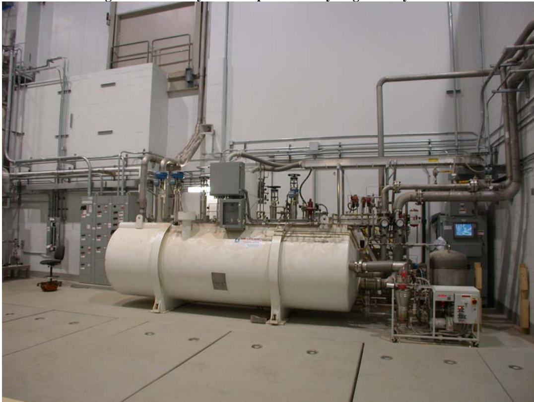
Fig. 5.2-37. Helium refrigerator cold box in RTBT location.
