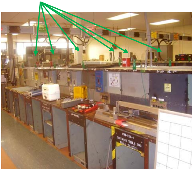
Green ground wires and clips, used for equipment grounding, were installed at four foot intervals along the workbenches.
