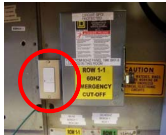
On complex circuits - GFCI Outlets were installed at the bench location to provide shock/fault protection to the bench circuit.
