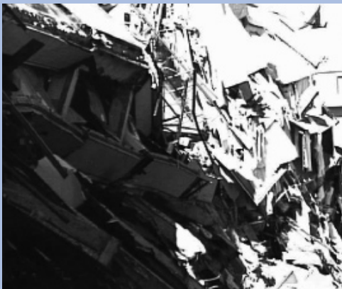
The New Orleans Riverwalk suffered extensive damage when it was struck by a bulk carrier vessel in 1996.
