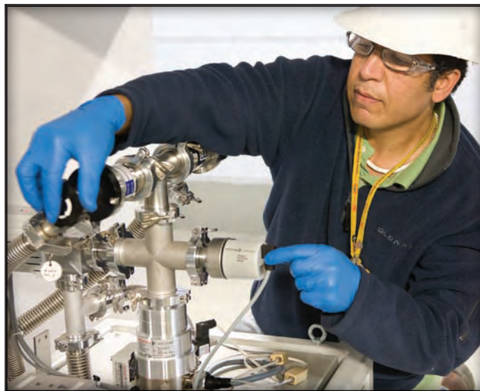
Saad Elorfi, Sample Environment Group, checks one of the main vacuum valves on the pumping station for the Backscattering Spectrometer to ensure that the systems are functioning properly.
