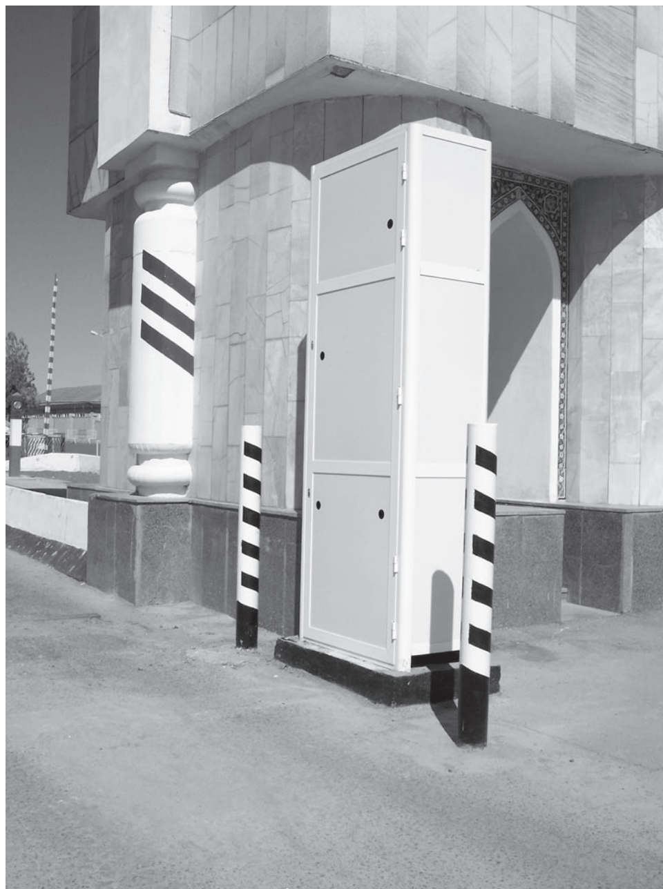
Figure 5: Radiation Portal Monitor in Uzbekistan with Heat Shield Enclosure
