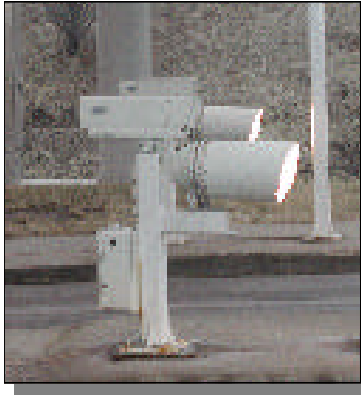
Exhibit 5-9 Illinois Tollway VES Equipment
