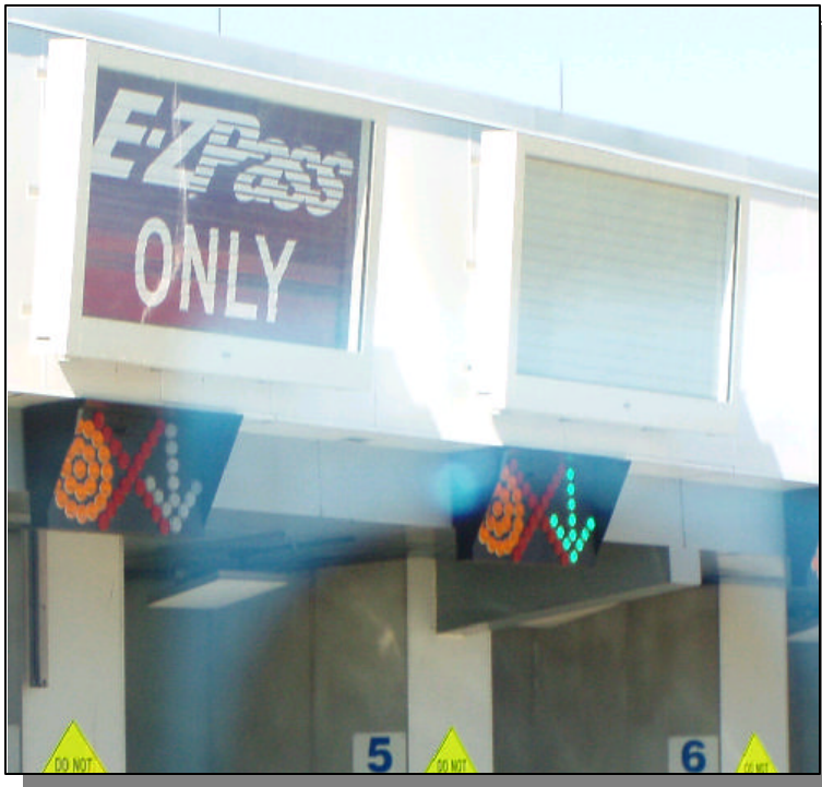
Exhibit 3-10 Delaware Memorial Bridge Toll Plaza Lane Use Signal & Changeable Lane Status Signs
