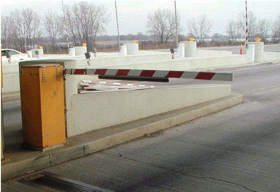
Exhibit 5-5 Indiana Toll Road Automatic Barrier Gate W/Gate Arm Impact Sensor
