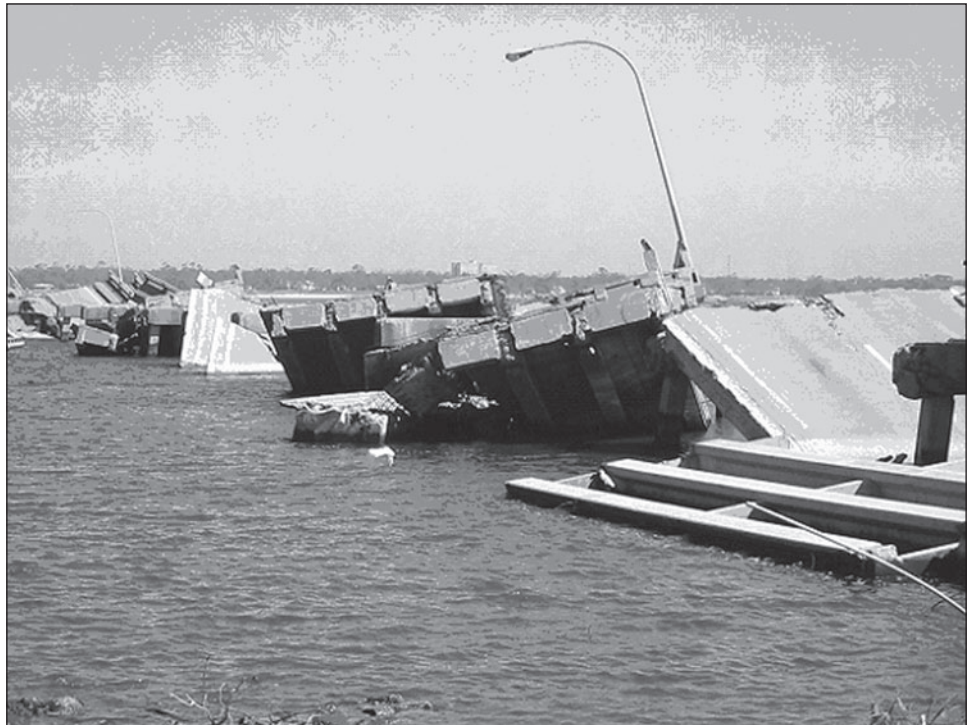
Figure 8: Damage to U.S. 90 Biloxi Bay Bridge
