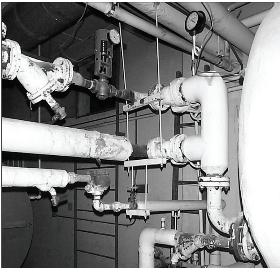
Figure 7: San Antonio Housing Authority—Corroded Heating and Air-Conditioning Pipes
