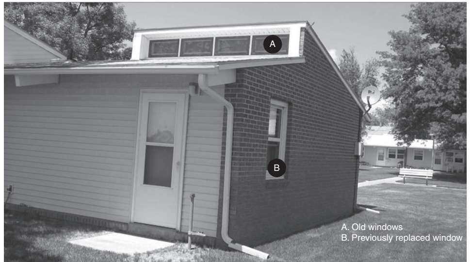
Figure 4: One Public Housing Unit at the Kersey, Colorado Housing Authority Before New Energy-Efficient Windows Were Installed (Upper Windows)
