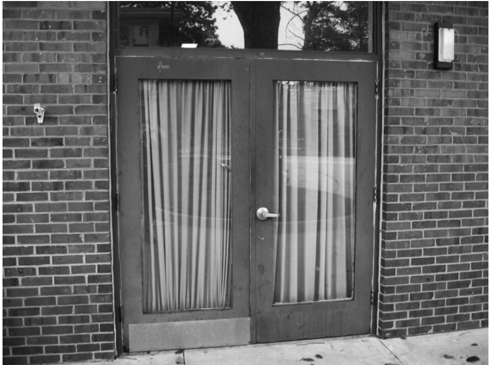
Figure 5: Candidate Door for Repair with Recovery Act Funds at the Kennedy Senior Housing Complex, Rahway New Jersey
