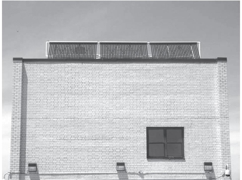
Figure 5: Installed Solar Panels on Top of a District of Columbia Housing Authority Residential Building
