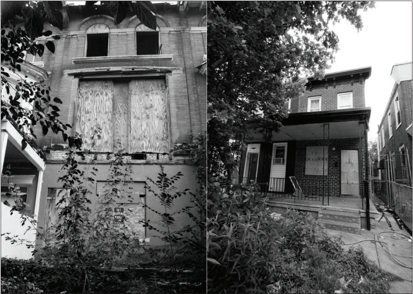
Figure 5: Two of the Vacant Units at Scattered Sites in Philadelphia, Pennsylvania, to Be Rehabilitated
