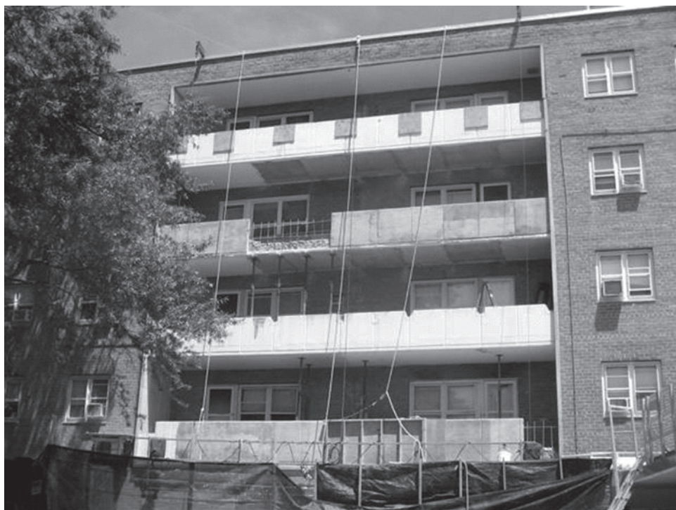
Figure 6: Balcony Rehabilitation Work at a District of Columbia Housing Authority Housing Complex
