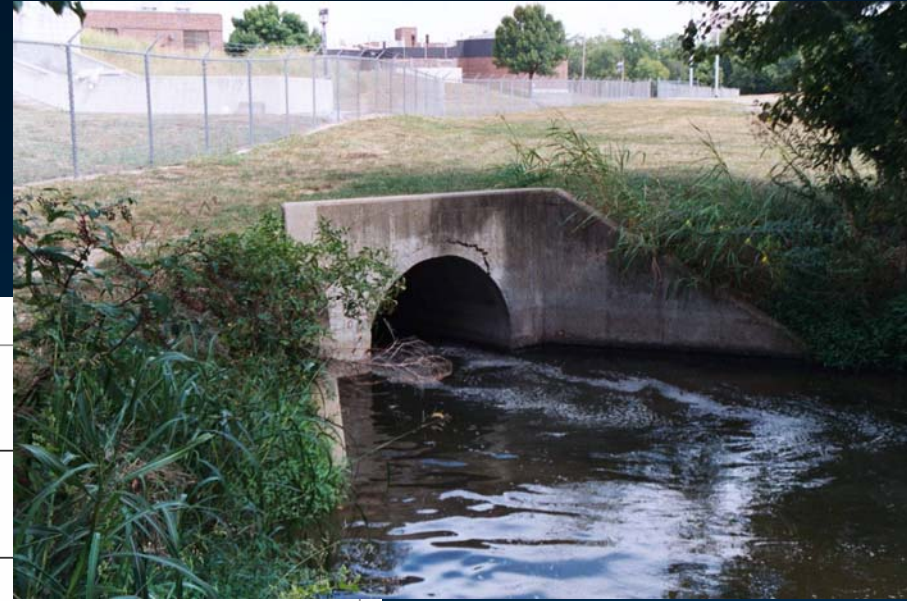
Indian Creek Middle Basin WWTF
