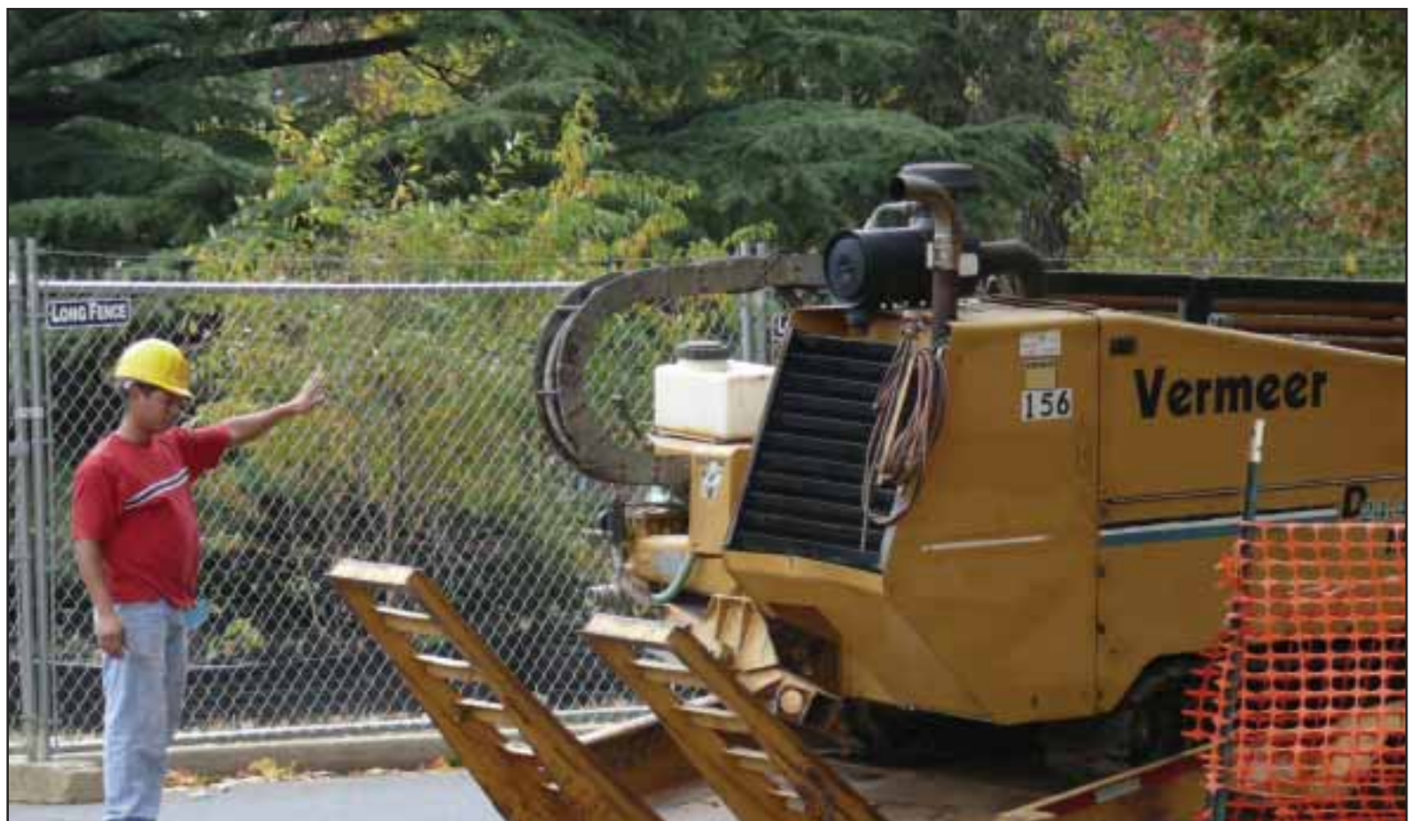
A worker directs placement of the trailer for offloading equipment. The renovation of the Lincoln Cottage is nearly complete. All residents are invited to an open house on Thursday, Dec. 6 at 1 p.m.
