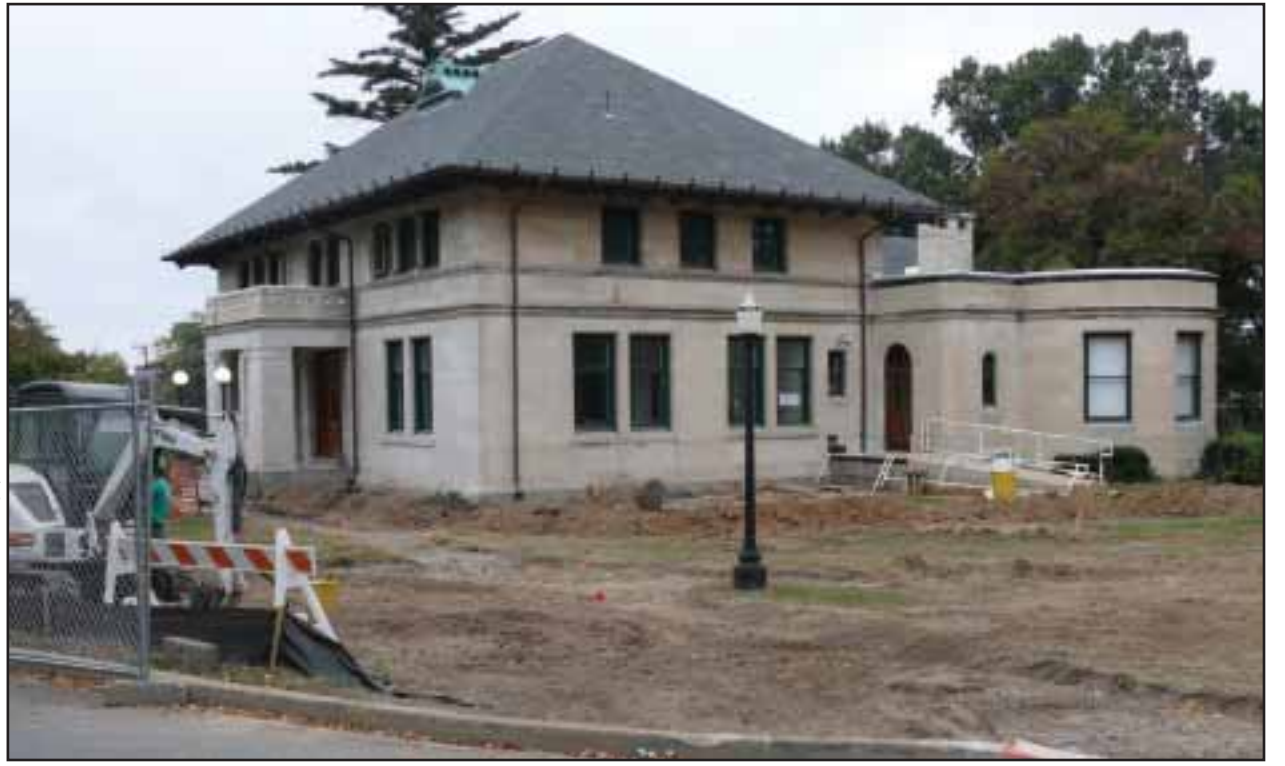
Work continues on President Lincoln's Cottage which is located on the AFRH campus. Managed by the National Trust for Historic Preservation, the Lincoln Cottage will be open to the public for tour on Feb. 8, 2008.
