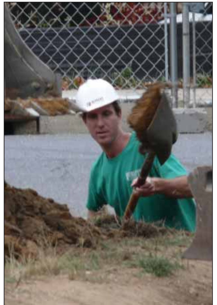
A worker shovels dirt in the area around the Lincoln Cottage. Landscaping of the area is underway.
