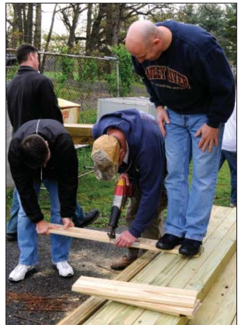
Right - Working together, the Coast Guard volunteers measure and cut lumber to be used in several projects down by the pond.
