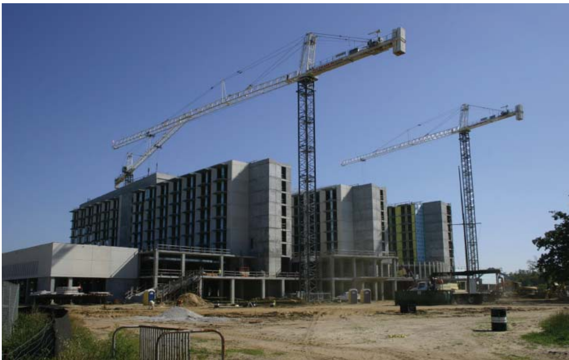
Construction of the new AFRH in Gulfport continues on schedule. See more photos of the progress on Page 3.
