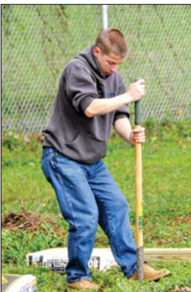
A volunteer uses a shovel to dig a post hole. In all, 21 posts were sunk around the pond to provide framework for a roped fence line.
