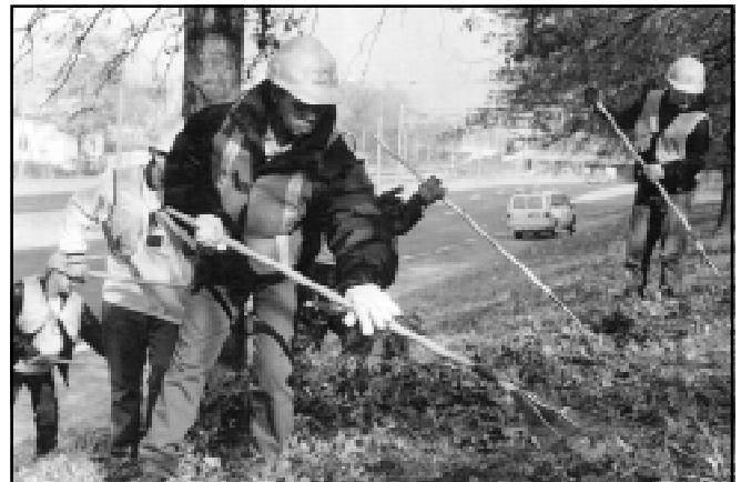
Work crew members wear proper safety gear while cleaning up roadside areas for the State Department of Transportation.
