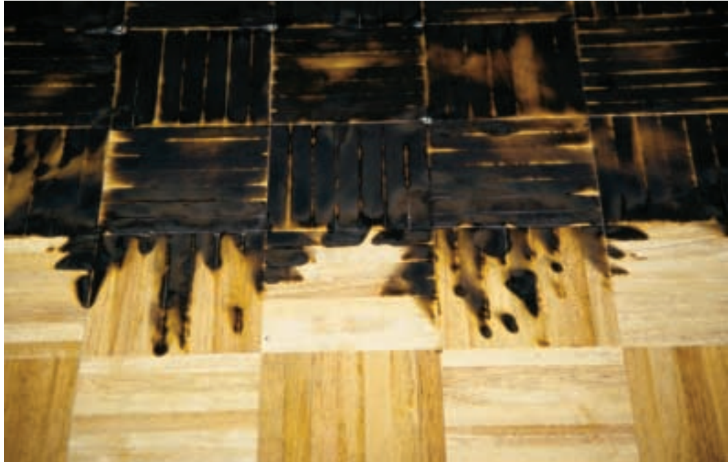
Figure 9. Closeup of gasoline spill fire burn pattern on wood parquet floor
