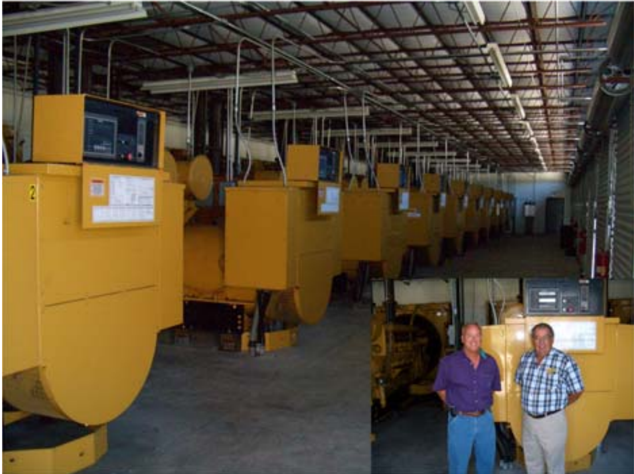
Figure 3 Powell Valley Distributed Generation with General Manager Randall Myers and Ronny Williams
