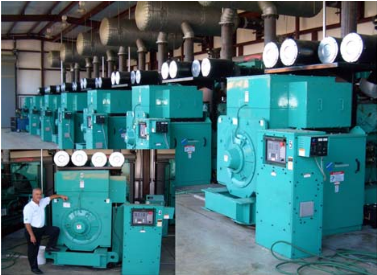
Figure 2 McMinnville Electric System Peaking Power Diesel Generator Sets with General Manager Rodney Boyd
