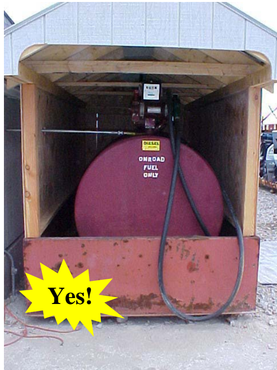
This gasoline storage tank is correctly installed inside secondary containment, sheltered by a roof, and surrounded by a concrete pad for controlling spills when dispensing gas from the storage tank into vehicles and equipment.
