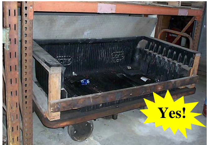
Clever idea! This simple battery storage box was made from an old truck bed.
