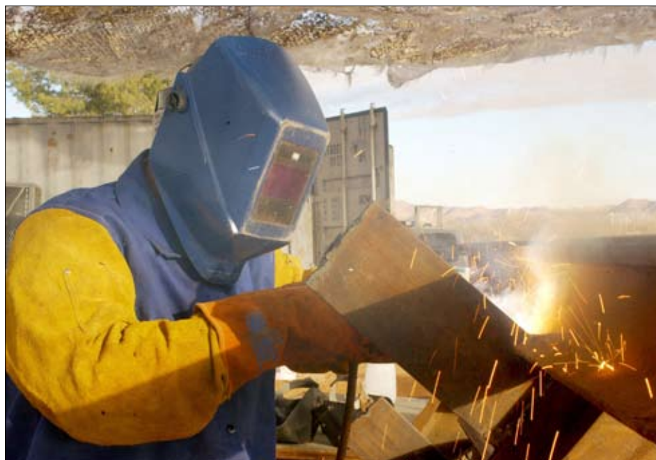
Sgt. Ross Willey of Portland, from E Co. (Civil Engineer Unit) 3rd Bn. 116th Cav., welds a railroad tie into place to create a vehicle barrier south of Sasabe, Ariz., Jan. 19. The barriers are used to prevent vehicles from illegally crossing the Arizona-Mexico border.
