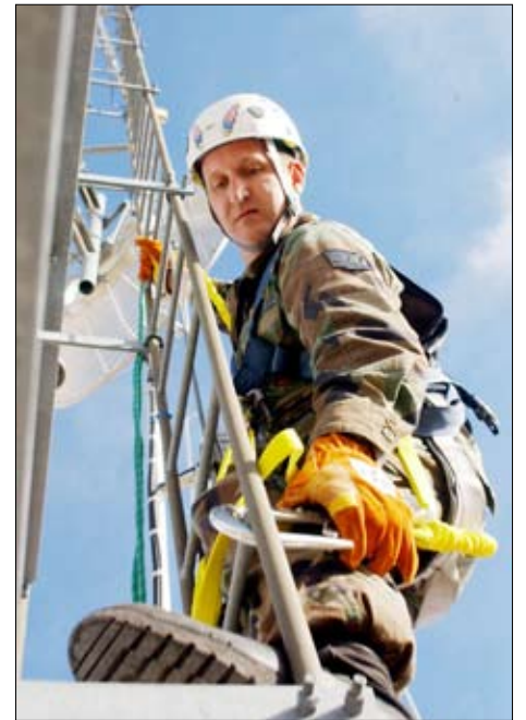
Tech. Sgt. Mark Quinn of Gresham, Ore., from 142nd FW Communications Flight, scales a communications tower near Tucson, Ariz., Jan. 18. Quinn is assigned to a Repeater Team responsible for upgrading communication systems for U.S. Customs and Border Patrol.
