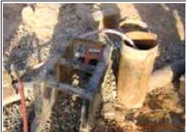
The small, ancient water pump in Dohela village, is in bad need of replacement, and their well needs to be dug deeper. (Photo courtesy of TF 2-116 Armor)
