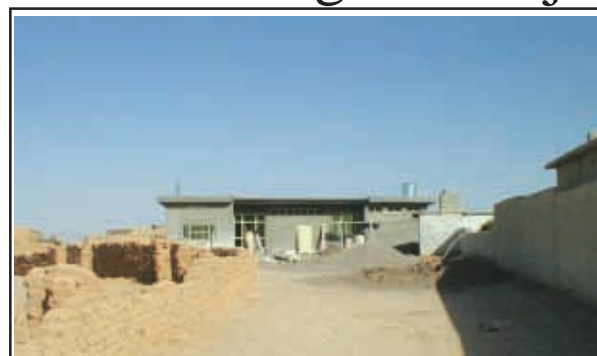
This photo of the front of the new Ranji, Iraq, clinic was taken July 20 by 116th Brigade Combat Team soldiers. The clinic is currently under construction, but is expected to dramatically improve both accessibility and quality of healthcare in the village.
