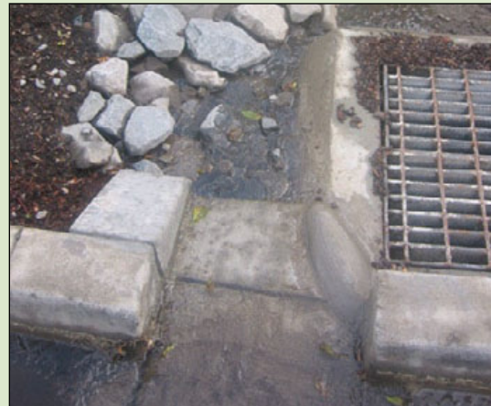
Figure C-15 Curb cut right next to the overflow.
