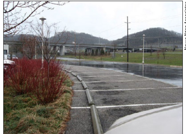
Figure 44. A pervious asphalt parking lot. The force applied by tires at turning, stopping, and starting locations can be hard on the paving surface.
