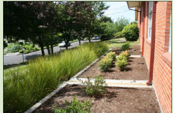
Figure D-7. A flow-through planter adjacent to an apartment complex in Portland, Oregon. This stormwater planter is completely lined to protect the building foundation from migrating water.
