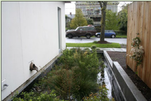
Figure D-6. An infiltration planter located away from the building foundation. Notice the surface conveyance of runoff to the planter by using a concrete runnel.
