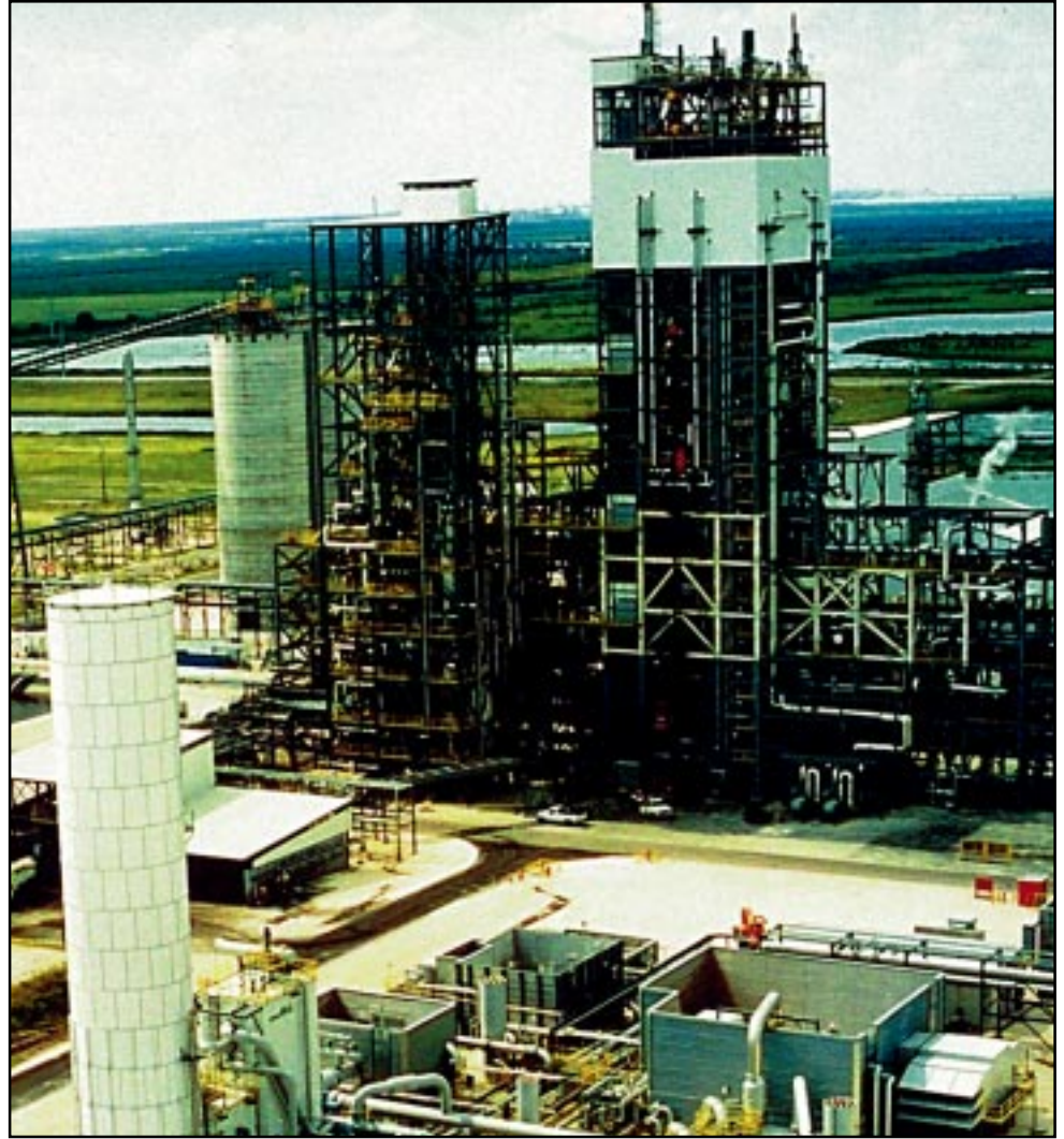
The Texaco gasifier is in the largest structure, which also contains the radiant syngas cooler. The hot gas cleanup system is installed in the smaller of the two large structures. In the foreground is the air separation unit.
