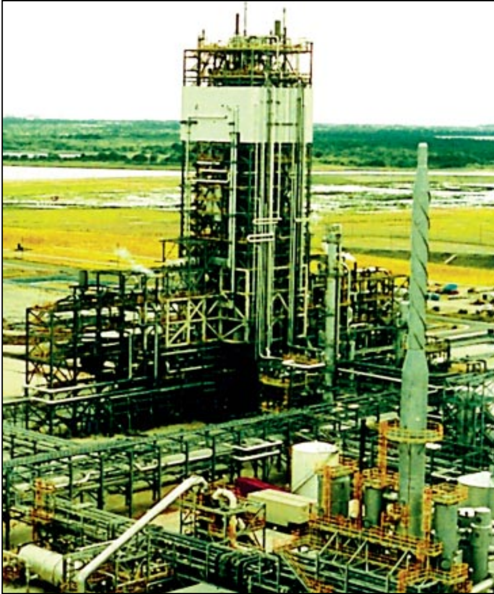
The sulfuric acid plant is located in the foreground and the gasifier and radiant syngas cooler are in the tall midground structure
