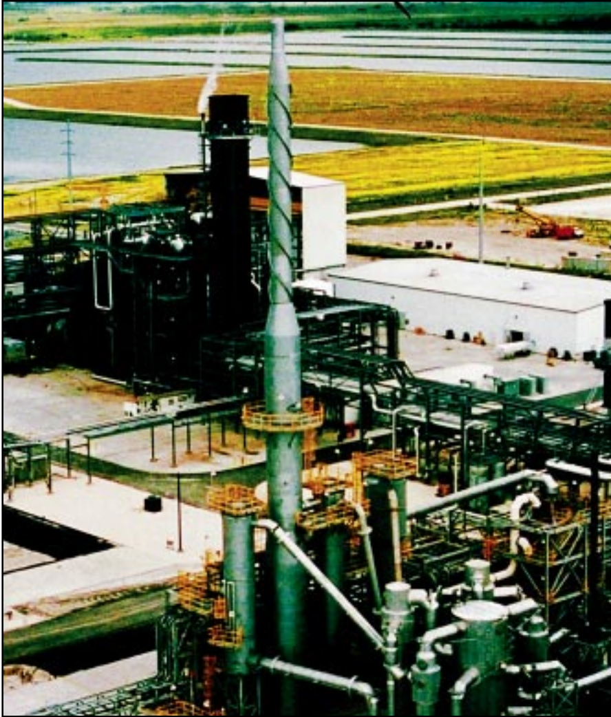
The sulfuric acid plant is in the foreground and the combined-cycle unit is in the background. The large black object (left center) is the heat recovery steam generator
