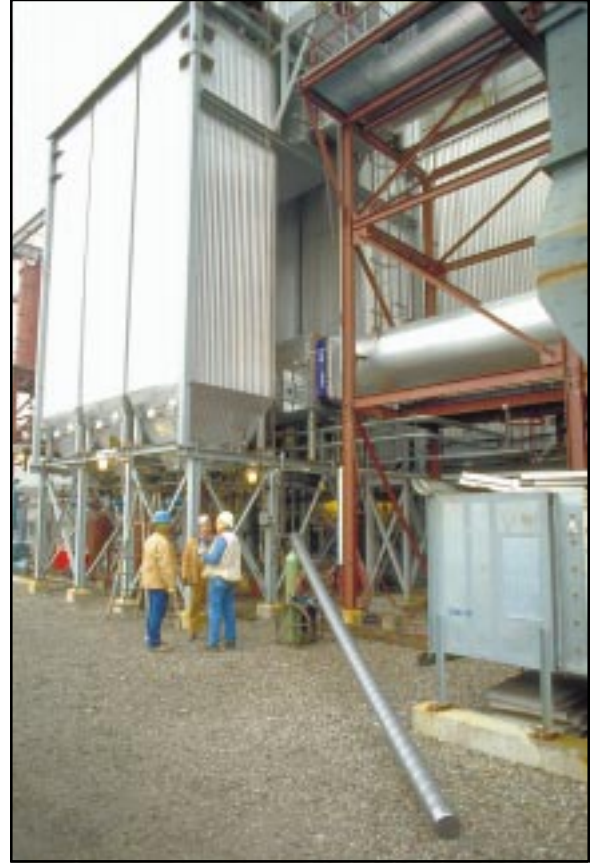
SNRB™ baghouse with catalyst holder tube ready for lifting into baghouse.
