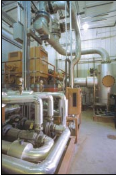
Urea injection system piping and compressor.
