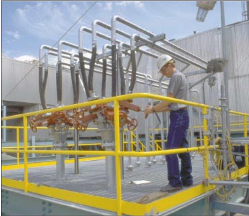
Sodium sorbent injection piping at Arapahoe Station.
