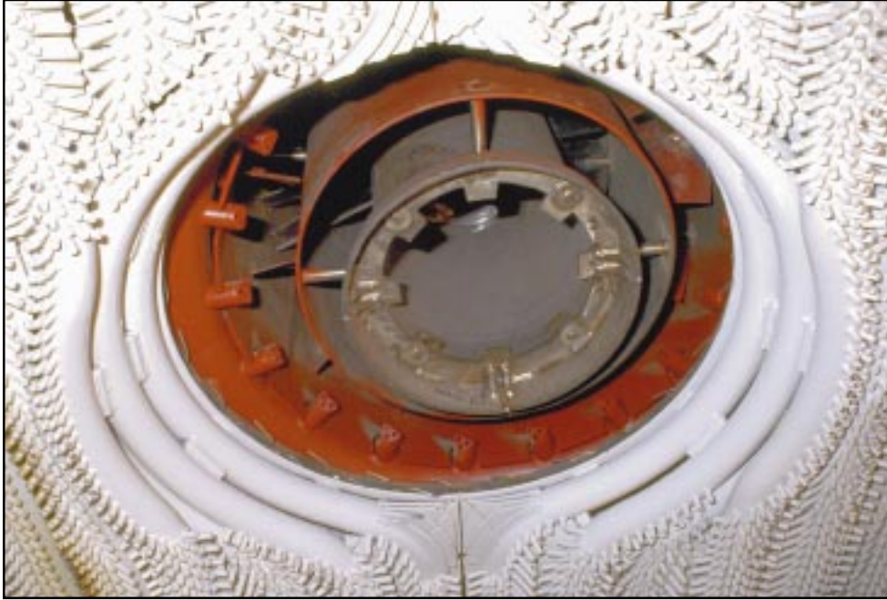
Tip of low-NOx burner installed on Unit 4 at Arapahoe Station.
