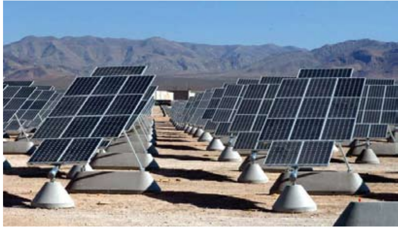
This 14-megawatt single axis, flat panel photovoltaic cell system is located at Nellis Air Force Base, Nevada. More than 72,000 solar panels occupy 140 acres – the largest solar photovoltaic system in North America.
