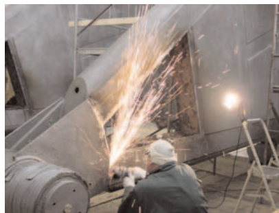
The culvert valve is being prepped for additional stiffener support (steel plates).
