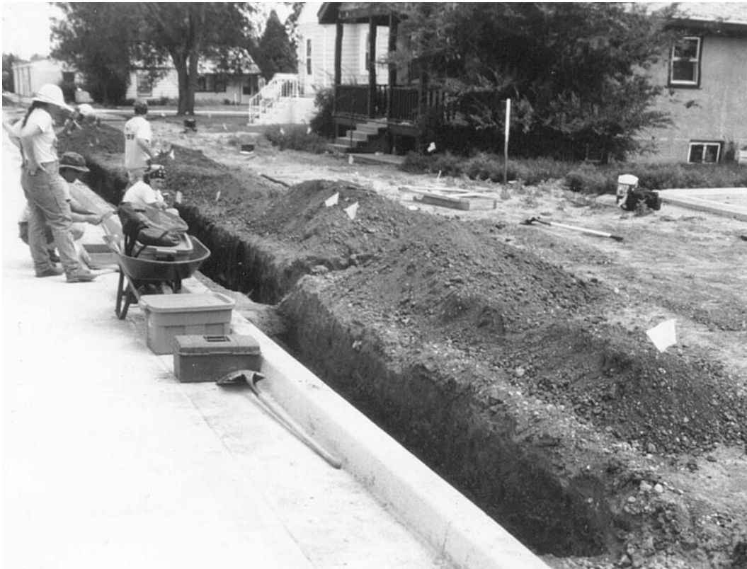
Figure 2.2. The sidewalk right of way on First Street NE.
