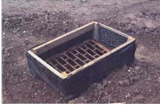
Silt Fence inlet protection structure
