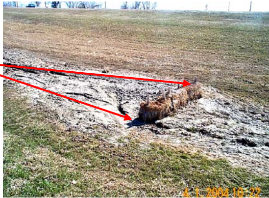
Improper installation of Bale Check
