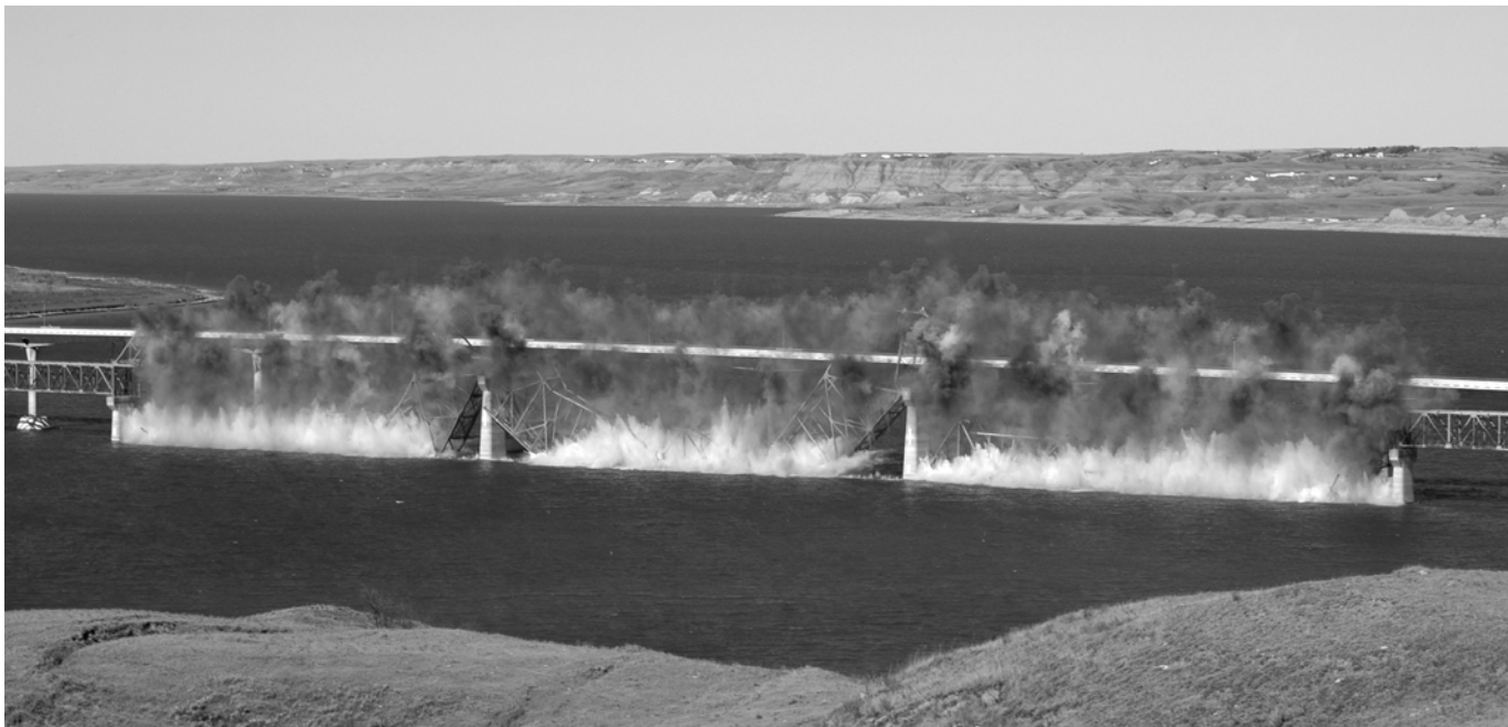
The the old Four Bears Bridge was demolished in October of 2005 after a new structure was built.
