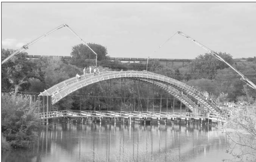
Concrete placement on the uniquely-designed Rainbow Arch Bridge in Valley City (see district report on left-hand page).
