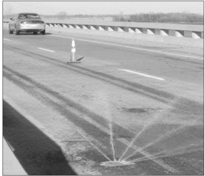
Anti-icing system at work on the Buxton Bridge deck.
