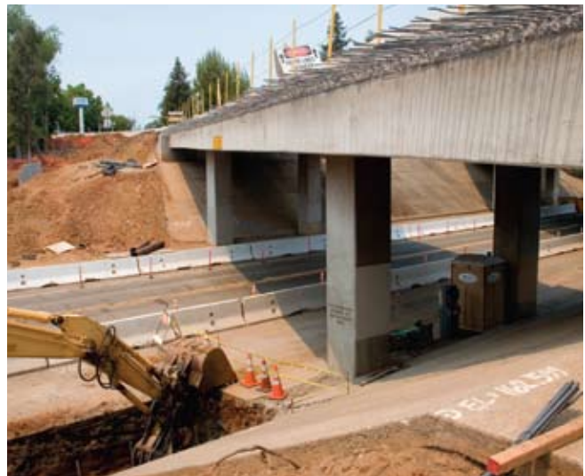
This photo shows the construction status of the Proposition 1B Dana to Downtown Redding congestion easing project as of July 9, 2008.
