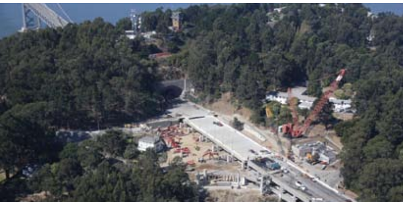
This aerial photo was taken September 4, 2007, after the Yerba Buena Viaduct section of the Bay Bridge was rolled into place.
