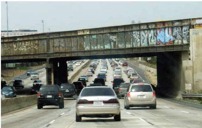
Caltrans cleaned up 12 million square feet of graffiti from the state highway system last year.
