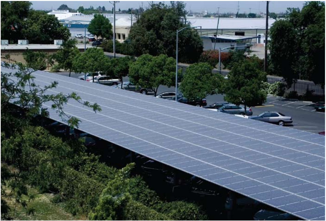
In an effort to be more environmentally friendly, Caltrans now uses this photovoltaic system to produce solar power for its Stockton offices.
