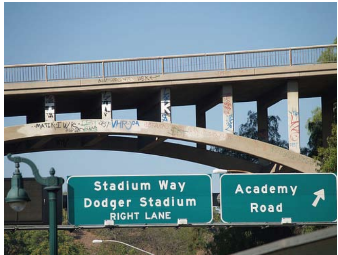
Graffiti, as shown here in Los Angeles, is an expensive state-wide problem.
