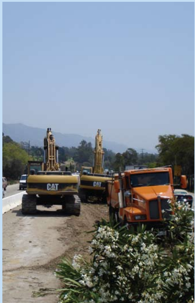
On July 16, 2008, crews cleared the median area for the Highway 101/Milpas Improvement Project in Santa Barbara.
