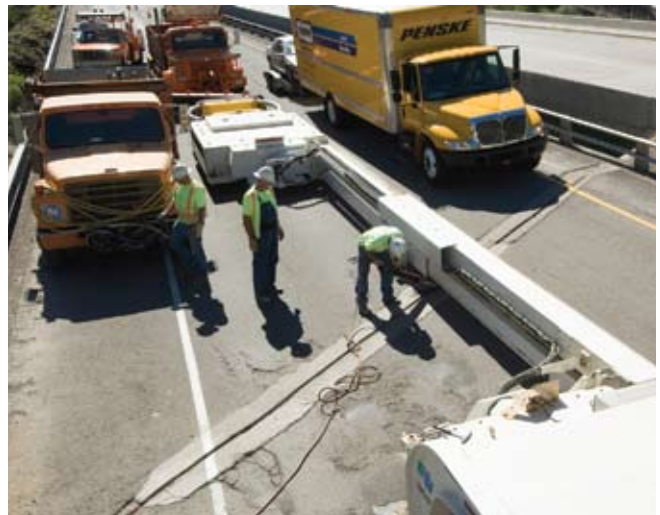
The Balsi Beam shields Caltrans maintenance workers from traffic while they repair a bridge expansion joint on Interstate 80, just west of the Nevada state line.
